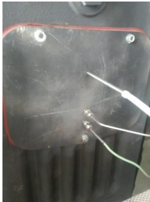
Figure 3-15. Temperature sensors in boiler
