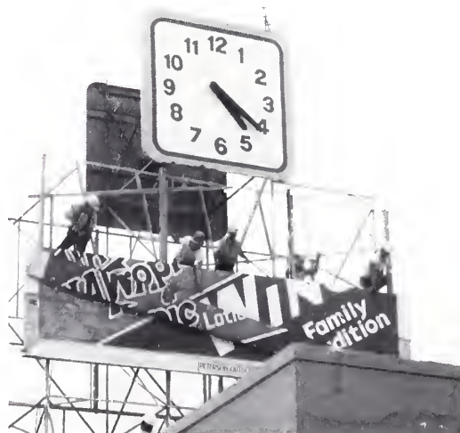
Ocean front billboards come down before the storm began.
