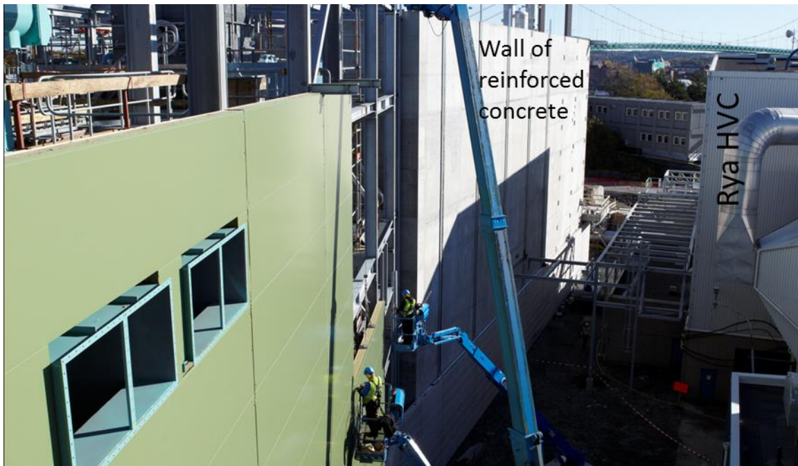
Figure 2.3: Illustrating the proximity to the neighboring plant Rya HVC and the constructed wall of reinforced concrete.
