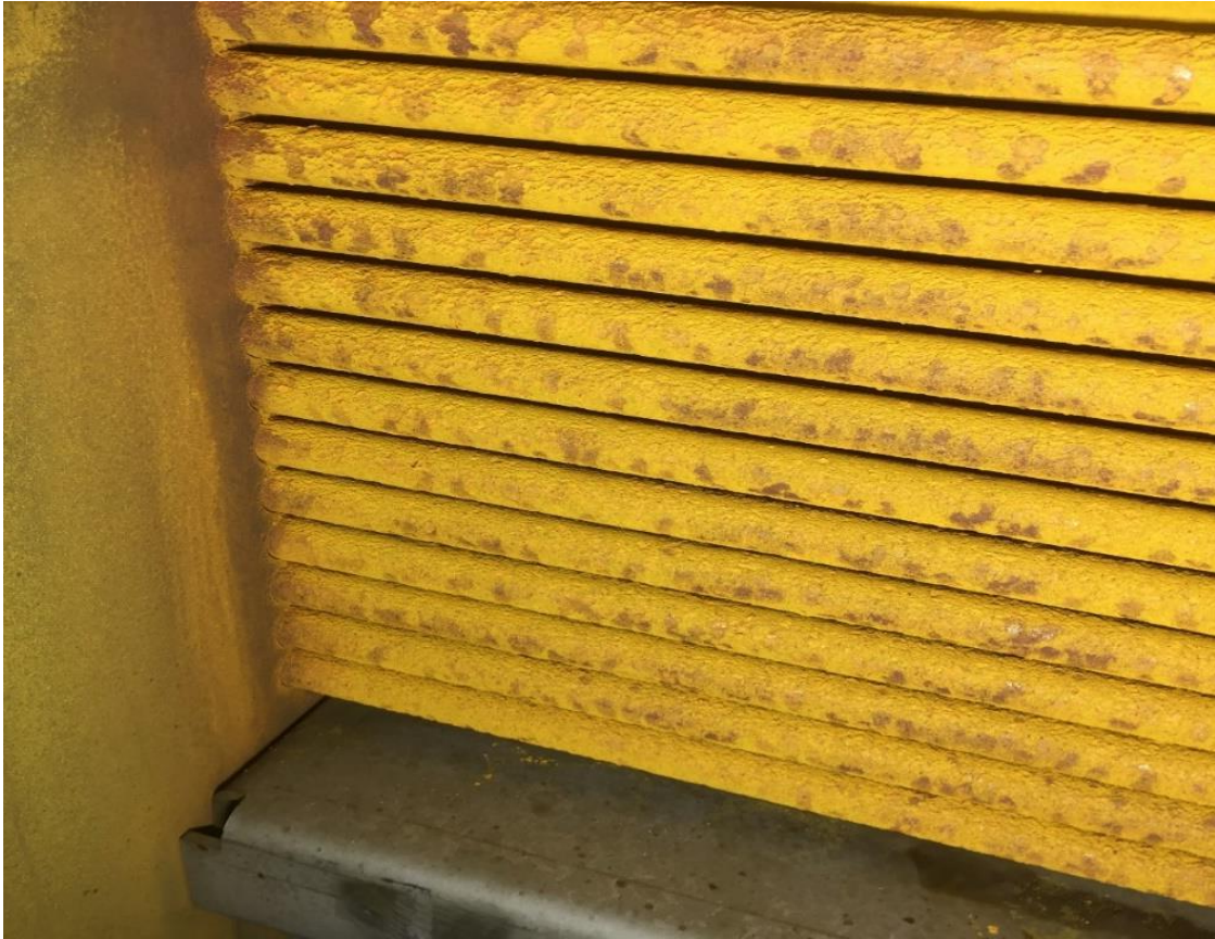
Figure 3.11: Deposits of tar components on the intercoolers in the product gas compressor.
