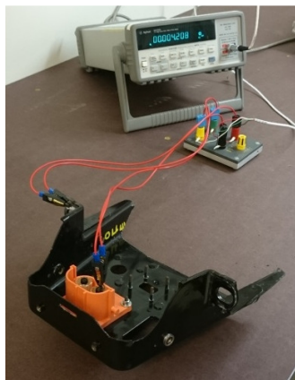
Figure 8.20 - Measurement of resistance between housing/chassis for battery and screen on DC connector.
