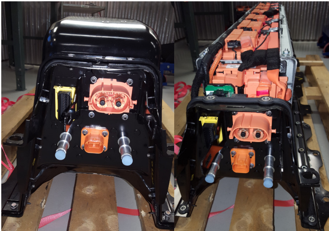
Figure 9.9 - Inert battery pack. The side with the CIDD (upper) and HVCH (lower) connector. With and without lid
