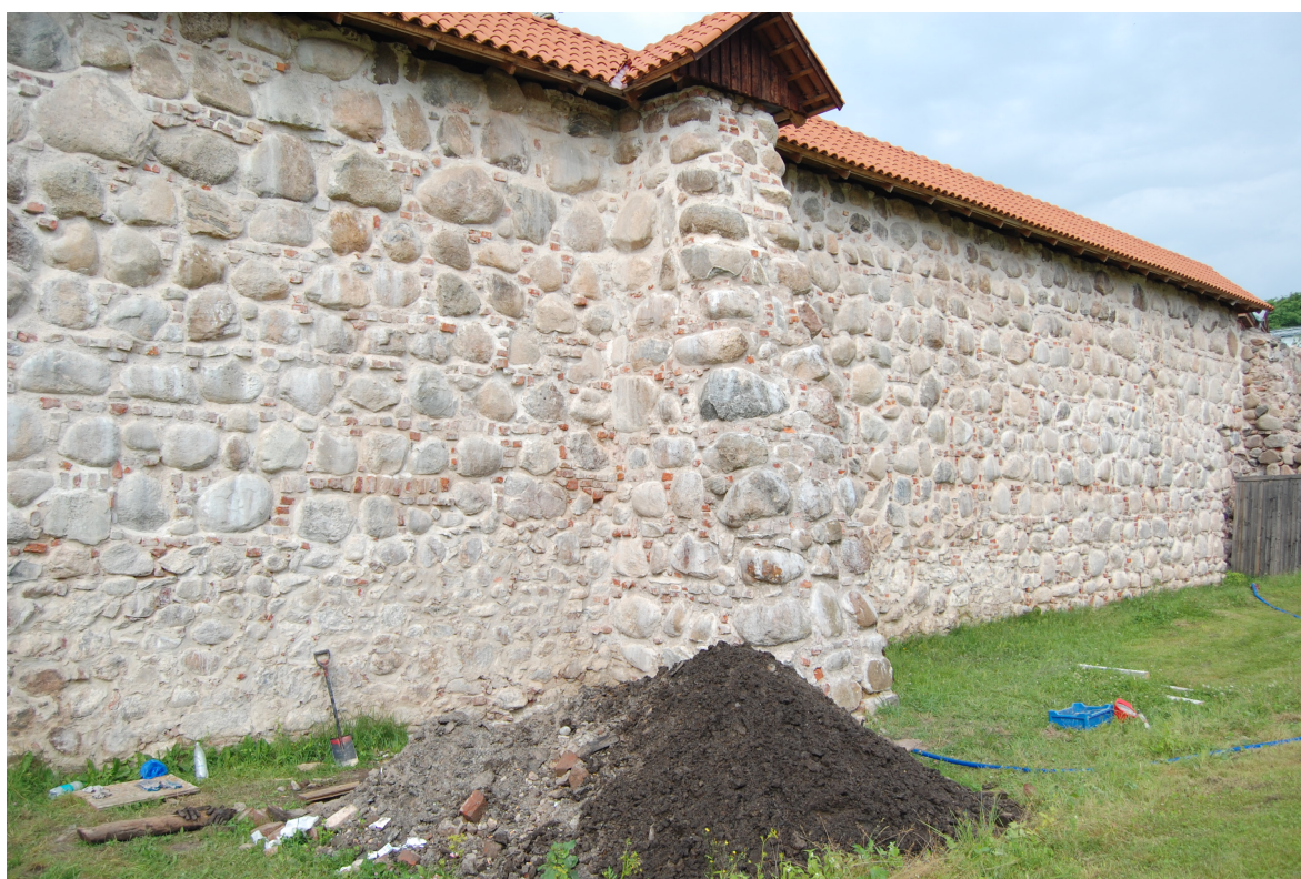
Figure 8. The renovated section of the town wall of Tartu in the riverside part of the town and the excavation pit in 2009. Photo by Rivo Bernotas.
