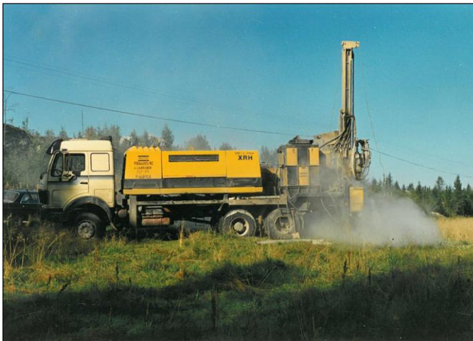
Fig. 36. DTH-drilling going on in the Tereniemi test well no. 931073 in the municipality of Viitasaari, Central Finland, in September of 1988. The final well depth was 43 m and Q=1,800 \text{ Lhr}^{-1} . Photo the author.
