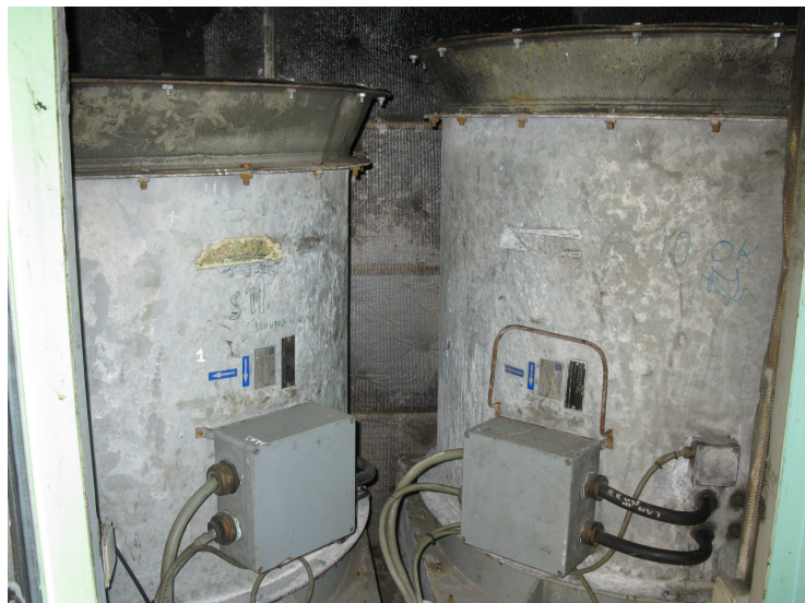
Picture 3. Main engine room ventilation fans
