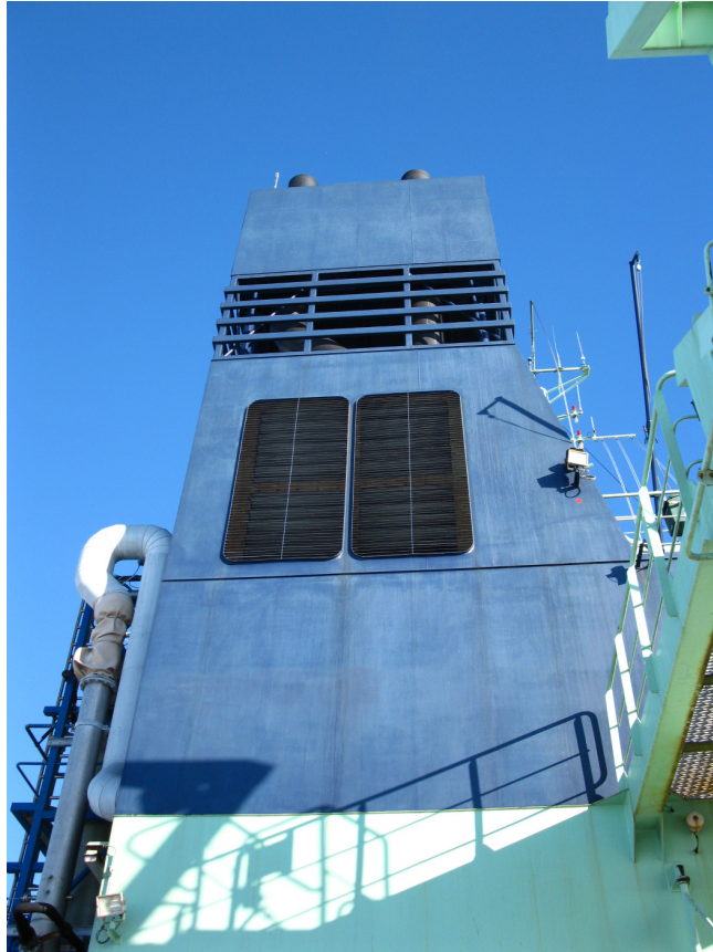
Picture 5. Ventilation air main exit
