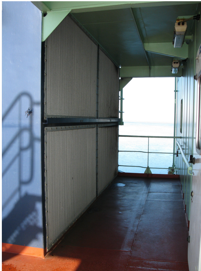
Picture 2. Air suction grills
