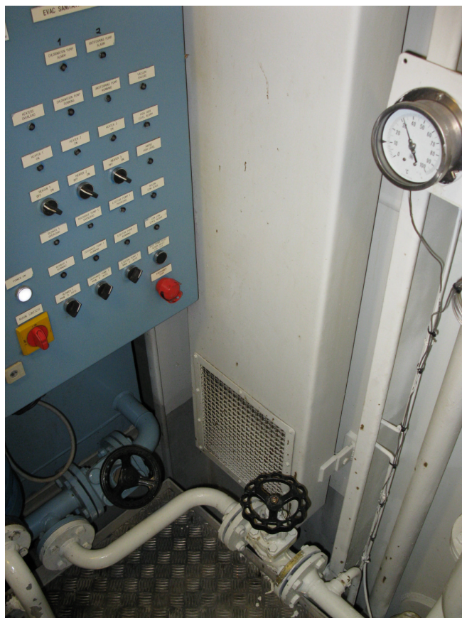
Picture 6. Bilge air suction
