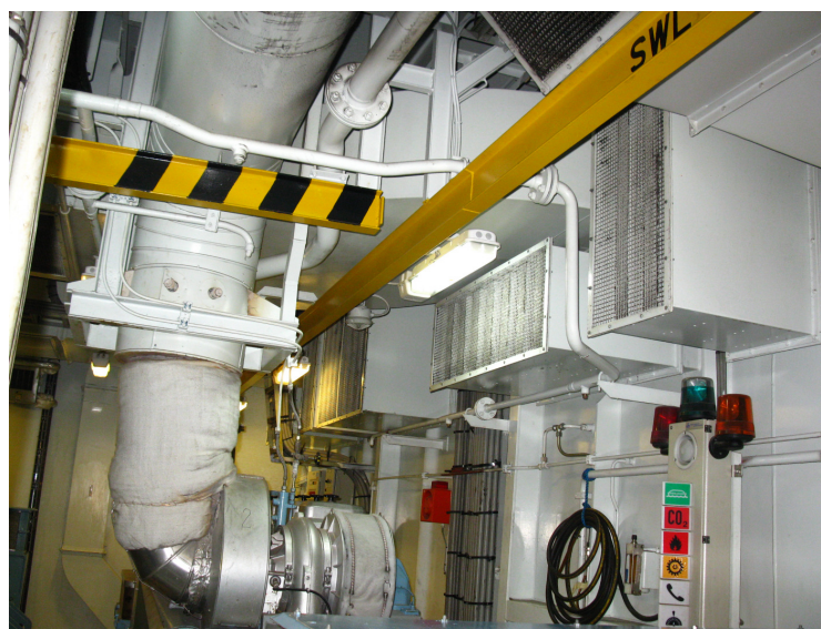
Picture 4. Ventilation air entrance ports from auxiliary engine room to main engine room
