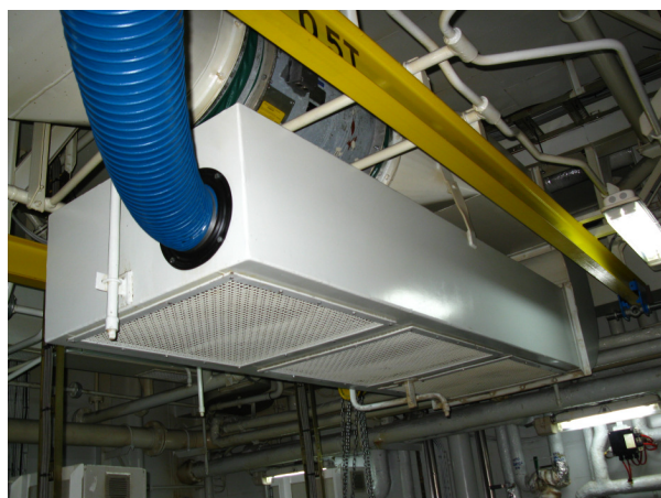
Picture 7. Separator room air exit grill
