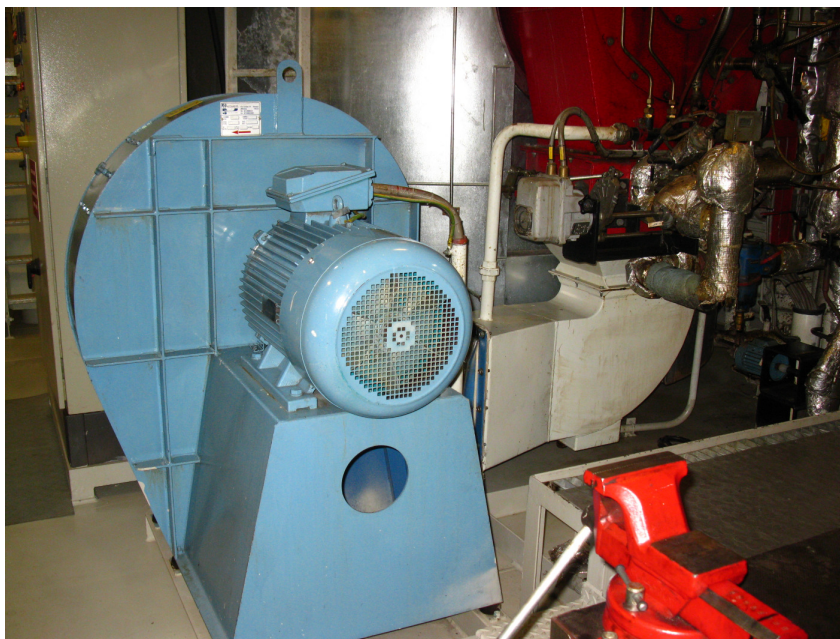
Picture 10. Steam boiler burning air fan
