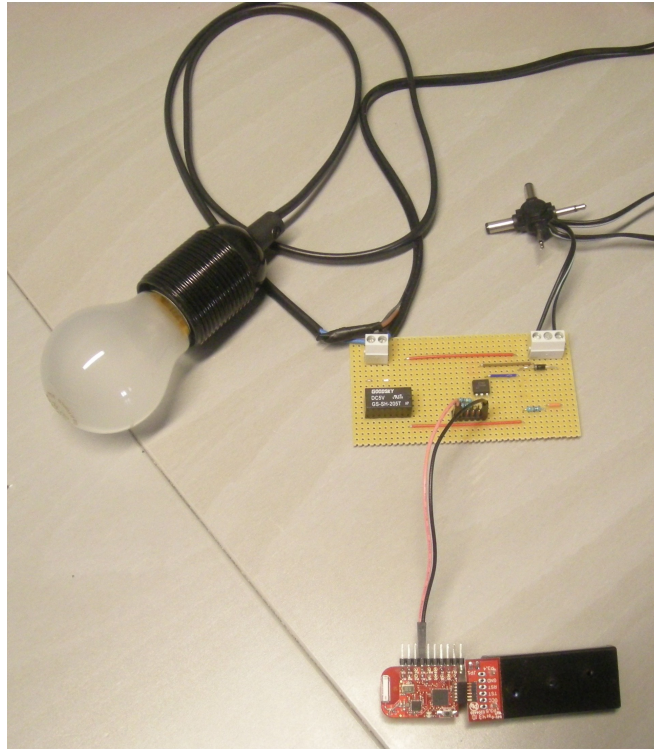
Figure 12. Lighting control board connected with the end device and the light bulb.
