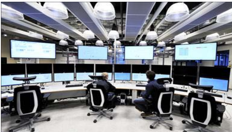
Figure 2. ABB data center in Västerås, Sweden (ABB 2012).
