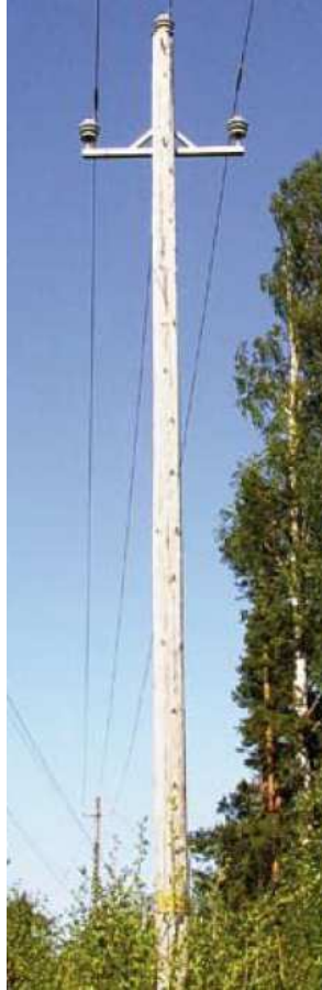
Figure 8. Typical tower type used in MV grid in Finland. (Turvatekniikan keskus 2007: 8)
