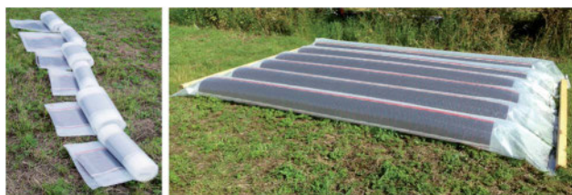
Fig. 4 Ground-based onshore solar cell installation with the rolled-up tubes prior to blow-up (left) and the final setup of six 3.4 m solar cell modules (right).
