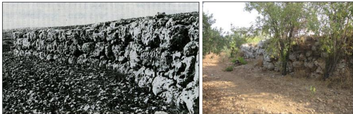
Fig. 7.15: The perimeter wall of the late IA village in Kh. Jarish, looking north, in 1968 (left; after Kochavi 1972b, Site 14) and in 2010 (right).
