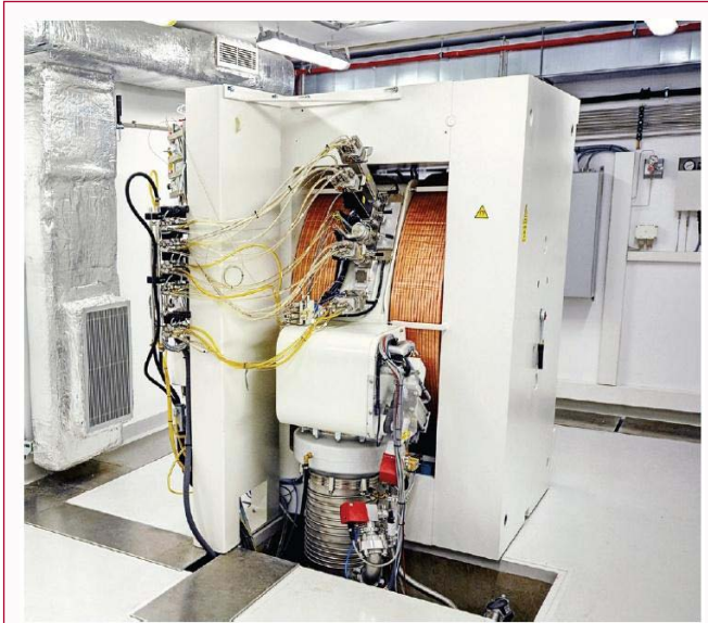
Figure 5: The PETtrace p/d cyclotron installed in its cave.
