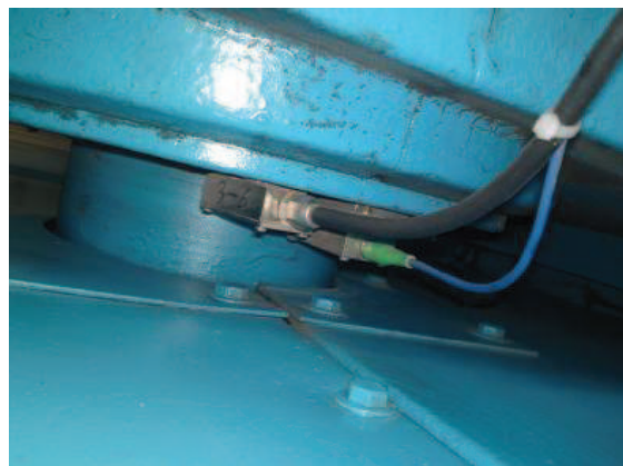
Figure 17 - Installation of machinery fault diagnosis system
