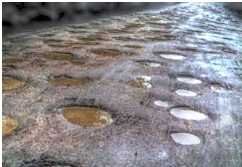
Figure 2.1: A road along which surface anomalies occur with a high frequency
