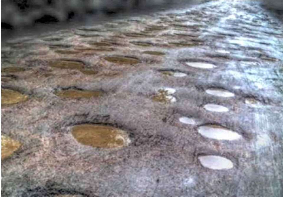
Figure 3.6: A stretch of bad road
