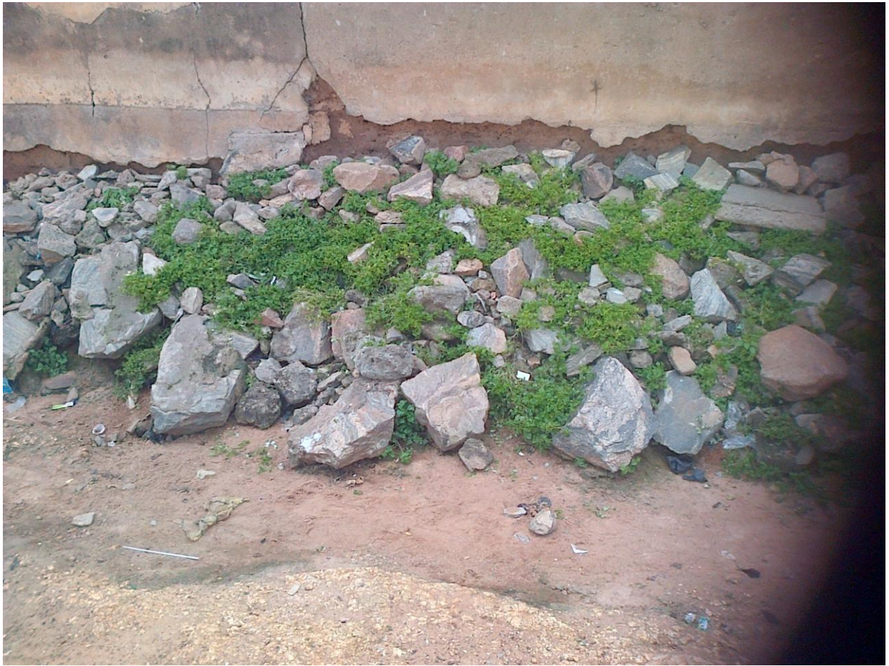
Plate 6: Local creativity in preventing further erosional impact on unpaved and ungreened open space around a building at Labo, Oranyan, Ibadan. Big boulders and rocks were used for this prevention. Consequently, green cover serves as prevention in addition to the stone used.
