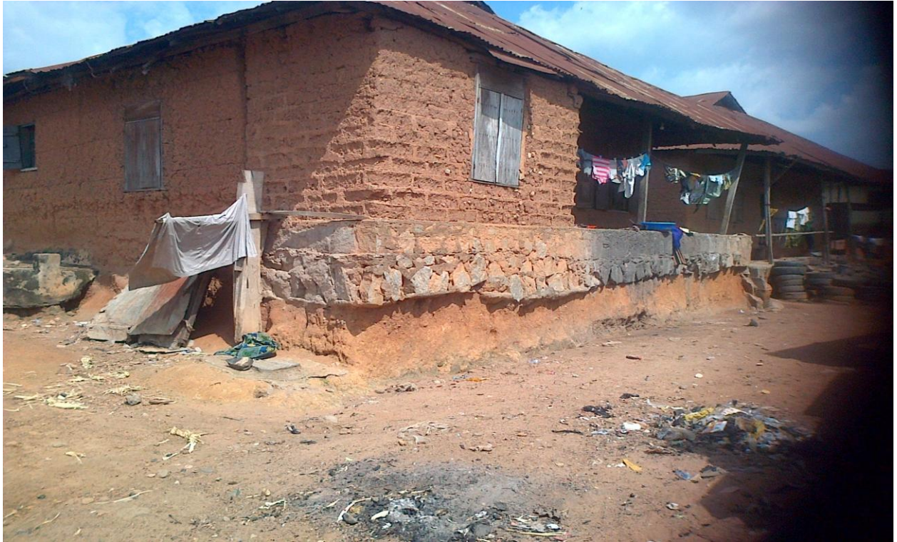
Plate 1: The Erosional effect on unpaved and ungreened open space around a building at Labo, Oranyan, Ibadan. The exposed foundation shows that large quantity of top soil had been washed away to the rivers and ocean.
