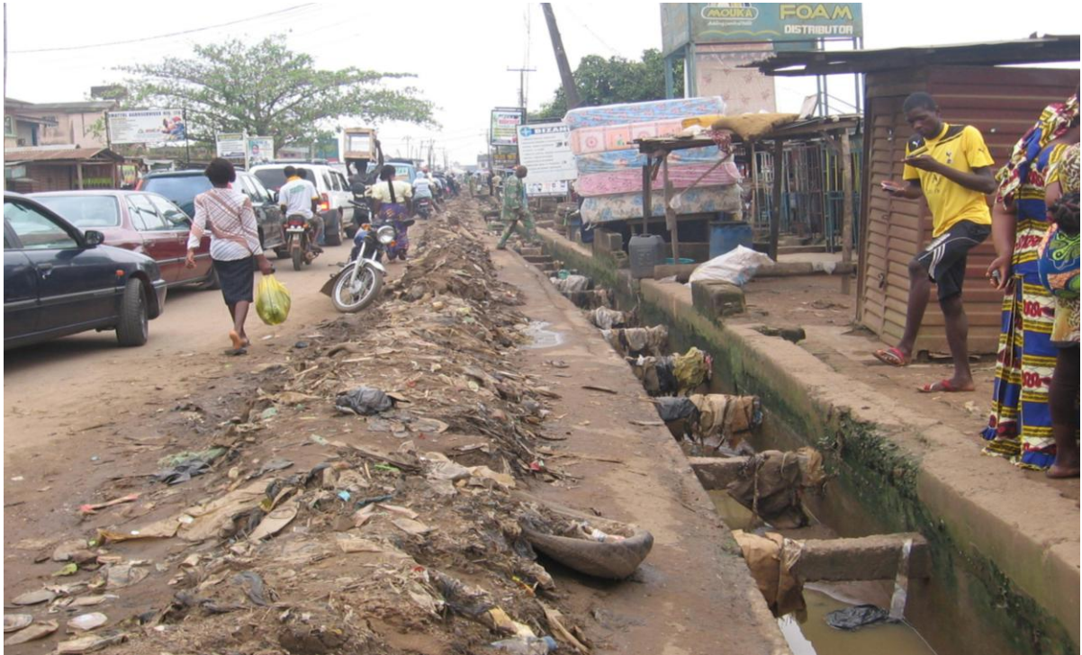
Plate 2: Large quantity of soil and other debris dug out of a drainage in Oju-Ore, Ota, a suburb of Lagos, confirming that unpaved and ungreened open space around buildings in the community generated large quantity of soil that were being washed away to the rivers and ocean.
