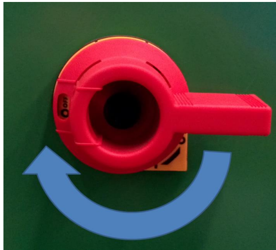
Figure 30: Main Wrapper Power
