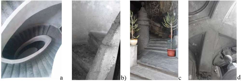
Figure 1: Palazzo Santoro, via Salita Capodimonte 10, Napoli [16]; b) small spiral staircase enclosed in a little room of the Sanfelice's Palace at Sanità district (Naples, Italy); c) The staircase in Sanfelice's Palace at Sanità district (Naples, Italy) object of the study [17]; d) the support vault.
