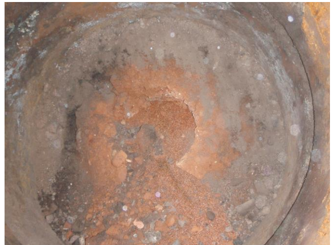
Figure 1. Smouldering remediation of coal tar in made ground. This is the top view into the excavation of a horizontal air injection experiment. The sharp transitions from remediated material in the centre to material that was unaffected by the process are evident, particularly on the left-hand side.
