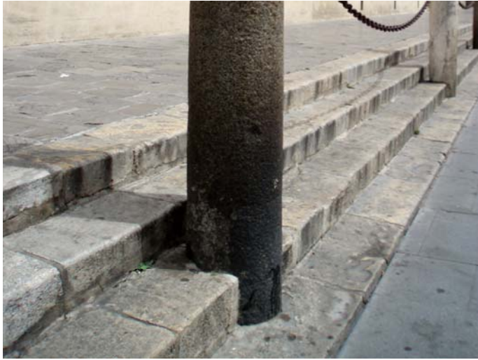
Figure 2: Granite column affected by crust, deposits and iron spots.
