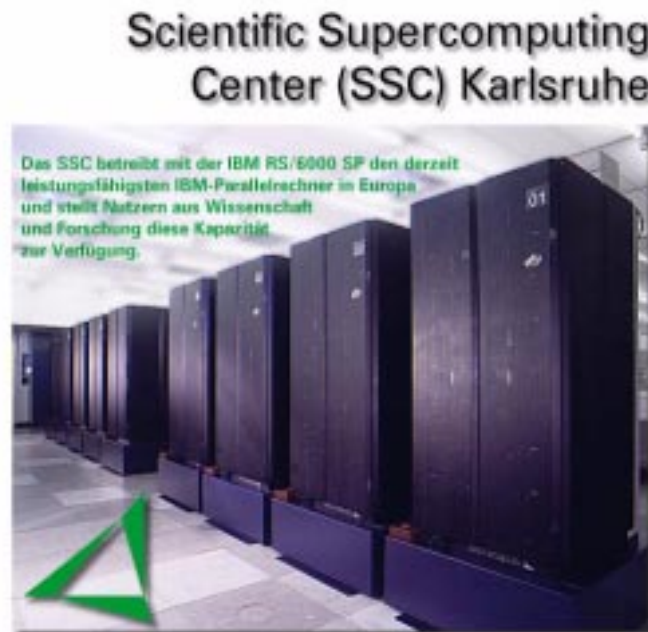
Figure 7: Scientific Supercomputing Center (SSC) Karlsruhe
