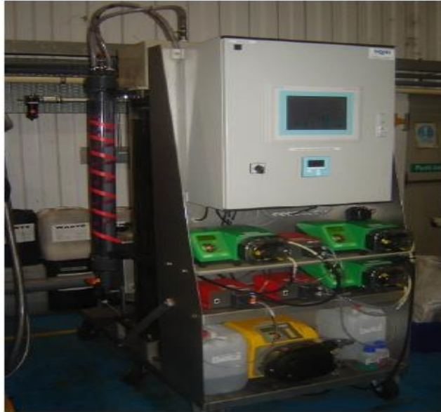
Figure 23. Expanded Granular Sludge Blanket reactor.
