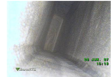
View into the cooling channel
