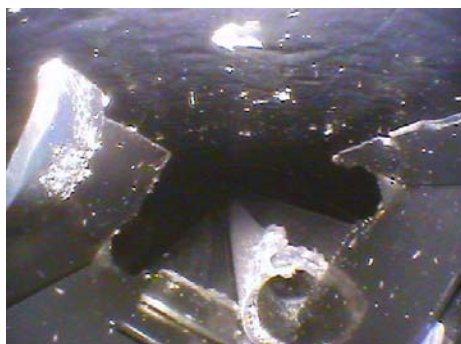
100 mm, top part of broken corner rod A, relocated and supported by grid spacer 2
