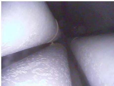
930 mm, spalling of thin oxide scales
