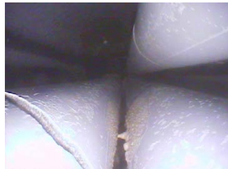
950 mm, circumferential cracks and negligible oxide spalling
