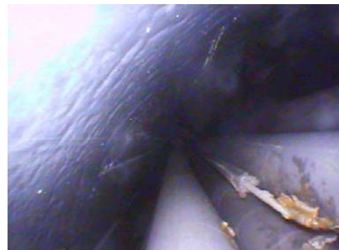
1070 mm, damaged TFS 14/14
