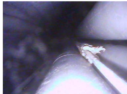
1000 mm, TFS 9/13 damaged sheathes
