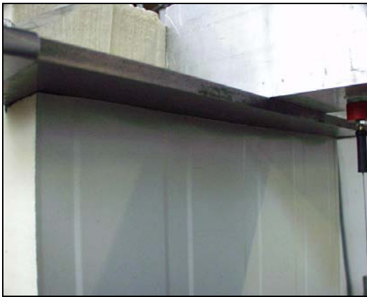
Failure of the stressed face
