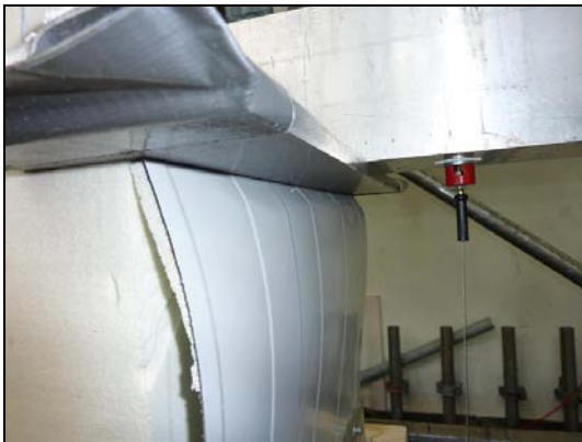
Failure of the stressed face
