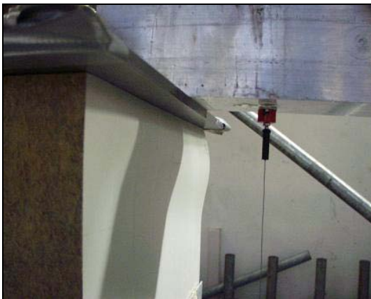
Failure of the stressed face
