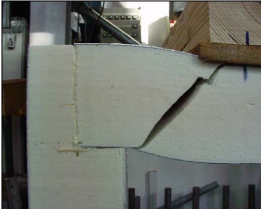
failure of the ceiling panel
