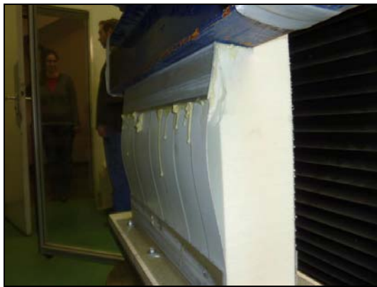
failure of the compressed face
