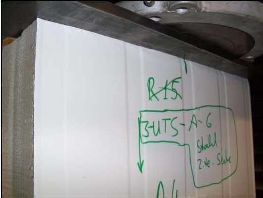
cripling of the stressed face
