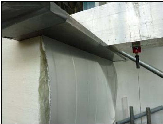
Failure of the stressed face
