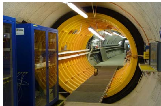
Fig. 2: The mega-packer system of the CFM experiment at the GTS. The shear zone is sealed with resin layer and surface packers are installed at outflow points on shear zone intersection. Pressurised water in annulus provides mechanical support to resin layer to counteract hydraulic head in the shear zone.
