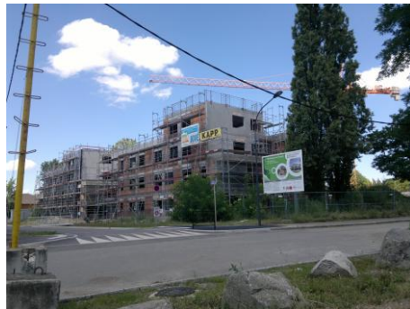
Figure 81 New constructions at rue du Fraternité on the site of the former ‘420’ in July 2012
