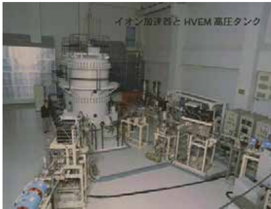
Ion beam irradiation facility in Hokkaido Univ.
