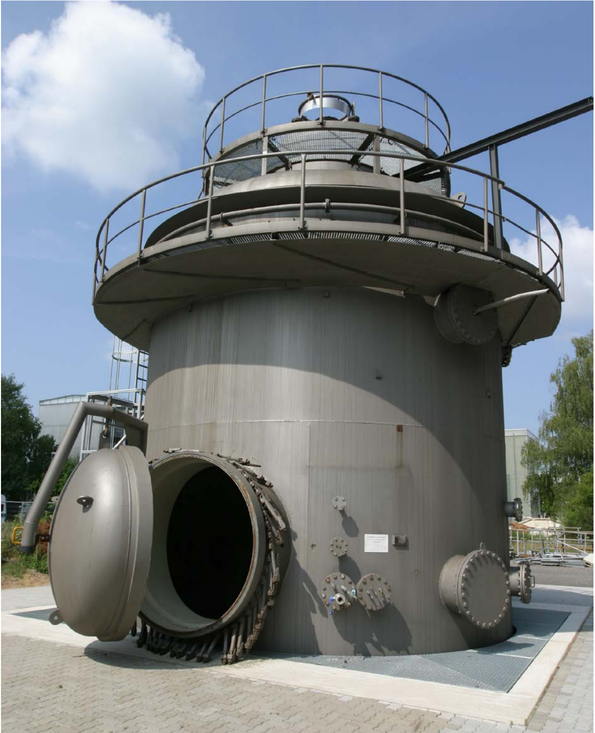
Fig. 2. Pressure vessel A2 without insulation and heating equipment
