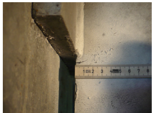
Crack caused by liquid metal embrittlement, found at the end of the half-plate weld
