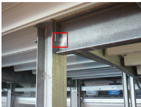
Zinc-coated steel girder with attached head plate in a multi-storey car park
