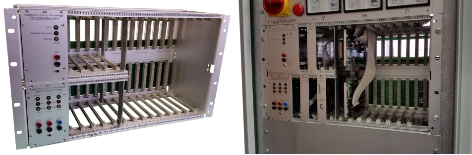
Fig. 3: Left: An empty subrack (19" / 6U) of the DSP-System. The backplane and the two power-supply units (5V, 15V, 24V) can be seen. Right: A partially populated subrack, already built into a control cabinet.
