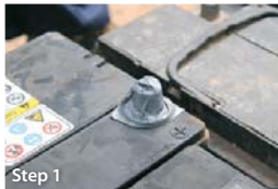
Step 1 Apply caps or isolation tape to the positive poles (+) of all batteries
