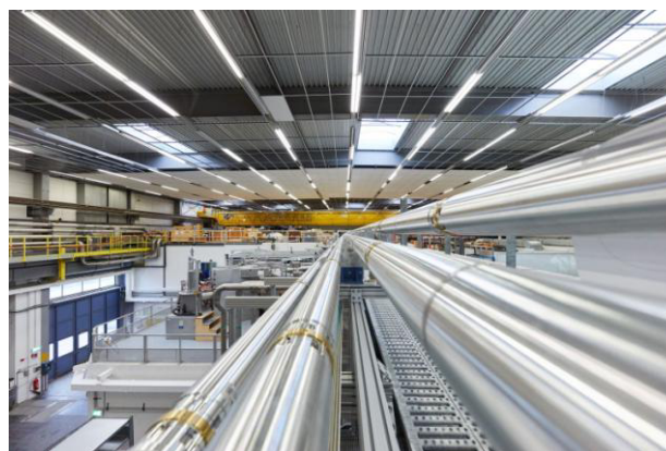
Fig. 1. View of the HE11 waveguide transmission line at ASDEX Upgrade
