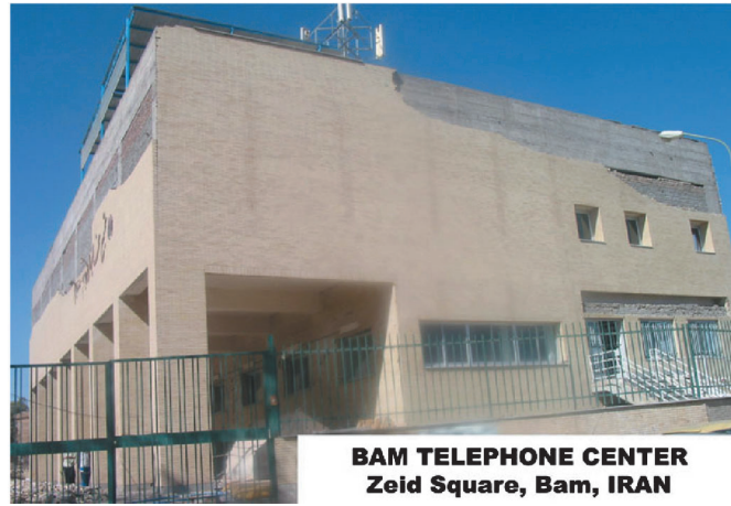
Fig. 1. Bam telephone center RC building after Dec. 2003 Earthquake, South and East sides.
