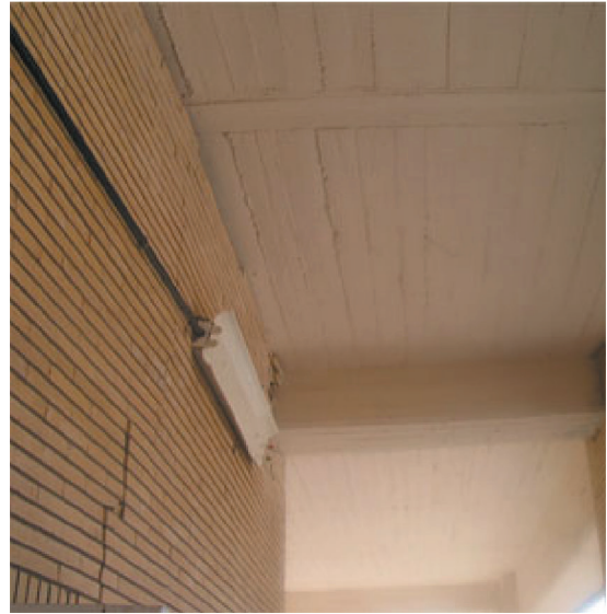
Fig. 28. Out of frame walls parallel to axis 1 between axis C and D, ground floor, with the maximum drift ratio of 0.9%.
