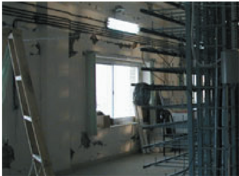
Fig. 27. Failure of the infill wall along the D axis in Fig. 4-b, Ground floor, with corresponding maximum drift ratio of 0.8%.
