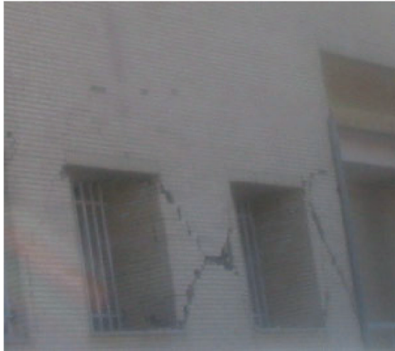
Fig. 24. Failure of the infill wall along the A axis in Fig. 4-b, between axis 6 and 7 in the ground floor, with corresponding maximum drift ratio of 0.9% from the analysis.
