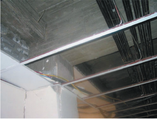
Fig. 21. A beam-column connection on the first floor of the Bam telephone center, which had no damage (about 1,000 m north of the strong motion station).
