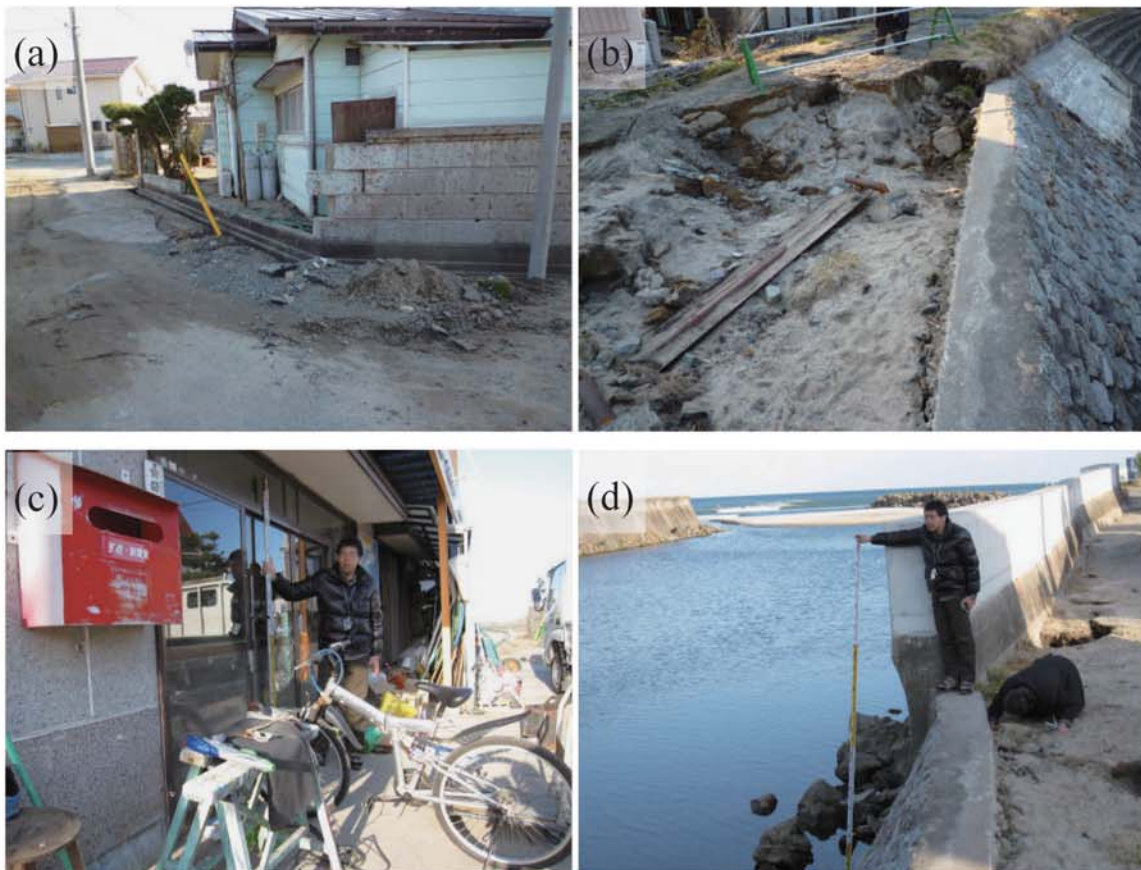
Fig. A252. (a)-(b) Damage at the side of the Sekine River in Hizencho. (c) Watermark on windowpanes of entrance sliding doors of the sign factory Kibokogei at the riverside in Hizencho (0.73m above ground level, B11). (d) Measuring ground height at the survey point based on the water surface in the Sekine River.
