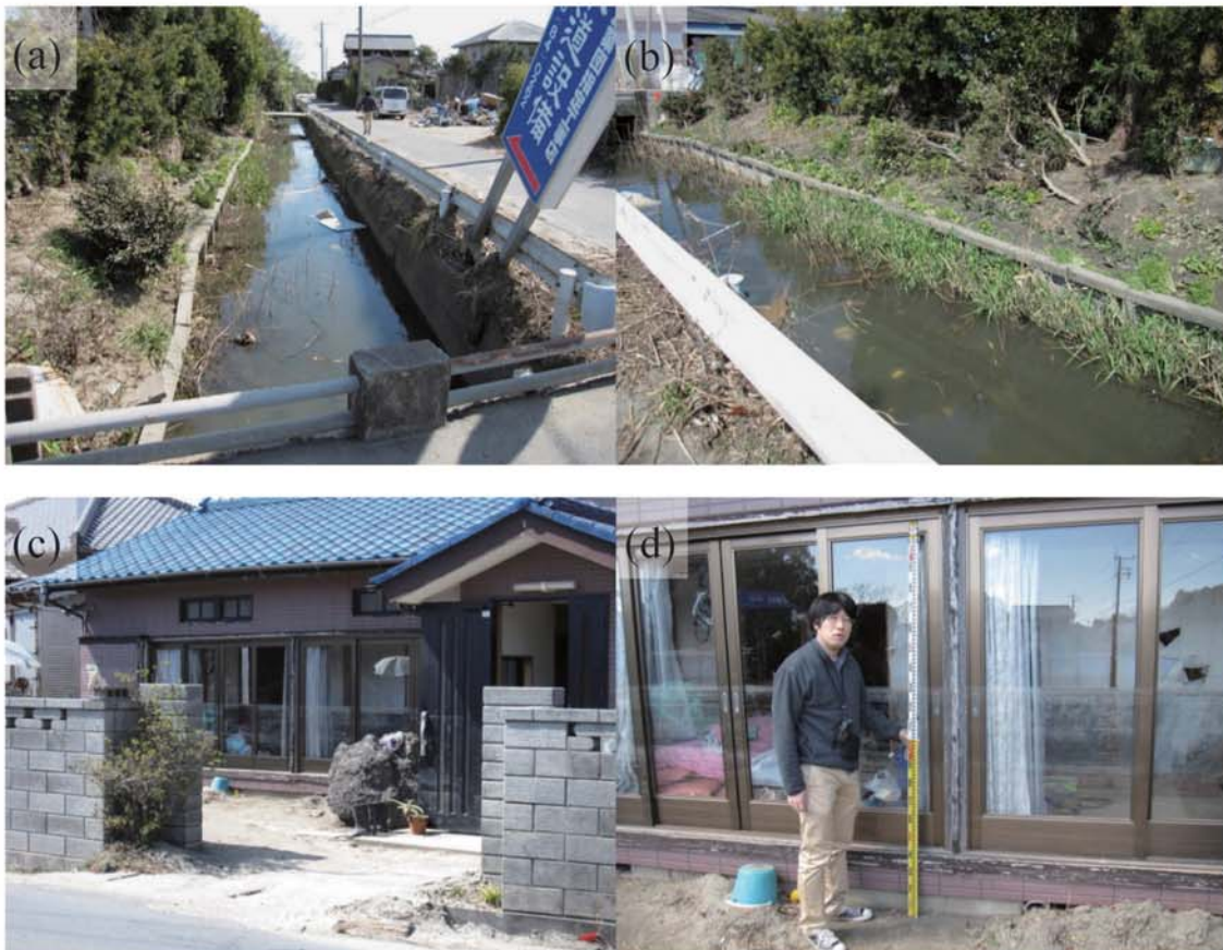
Fig. A312. (a)-(b) Damage due to tsunami run-up through the flume. (c)-(d) Watermark on windowpanes of Mr. Uchida's house (1.27 m above ground level; C14).
