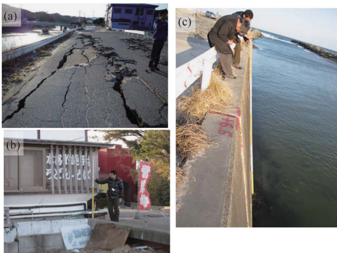
Fig. A254. (a) Liquefaction along the Hananuki River in Arakawa. (b) Tsunami trace survey point at the parking lot of the restaurant Sanukijyaya (B12). Tsunami inundated the top of the slope at the parking lot. (c) Measuring ground height at the survey point based on the water surface in the Hananuki River.
