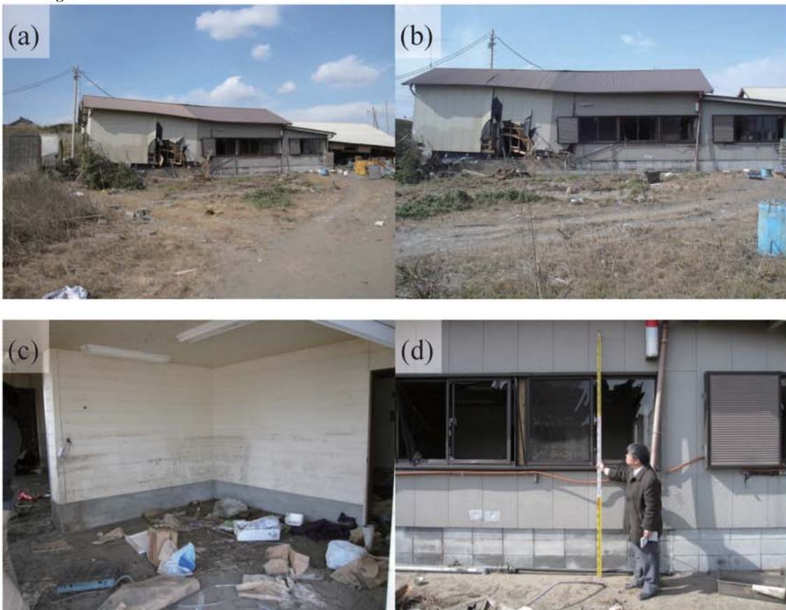
Fig. A302. (a)-(b) The building of a marine product-processing factory destroyed by the tsunami. (c)-(d) Watermark on a wall of a marine product-processing factory (1.94 m above ground level; C7).
