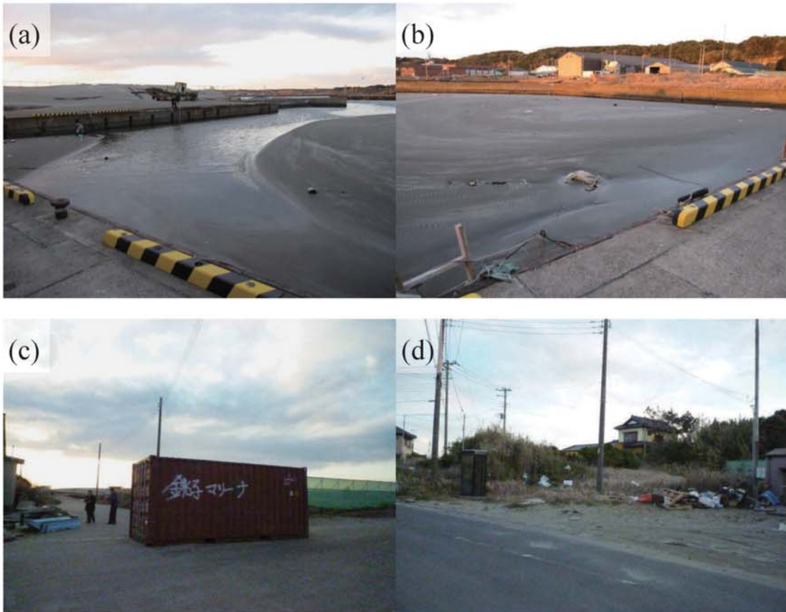
Fig. A294. (a)-(c) Inuwaka Fishing Port. (d) Watermark on a telephone box near Inuwaka Fishing Port (1.365 m above ground level; C2).
