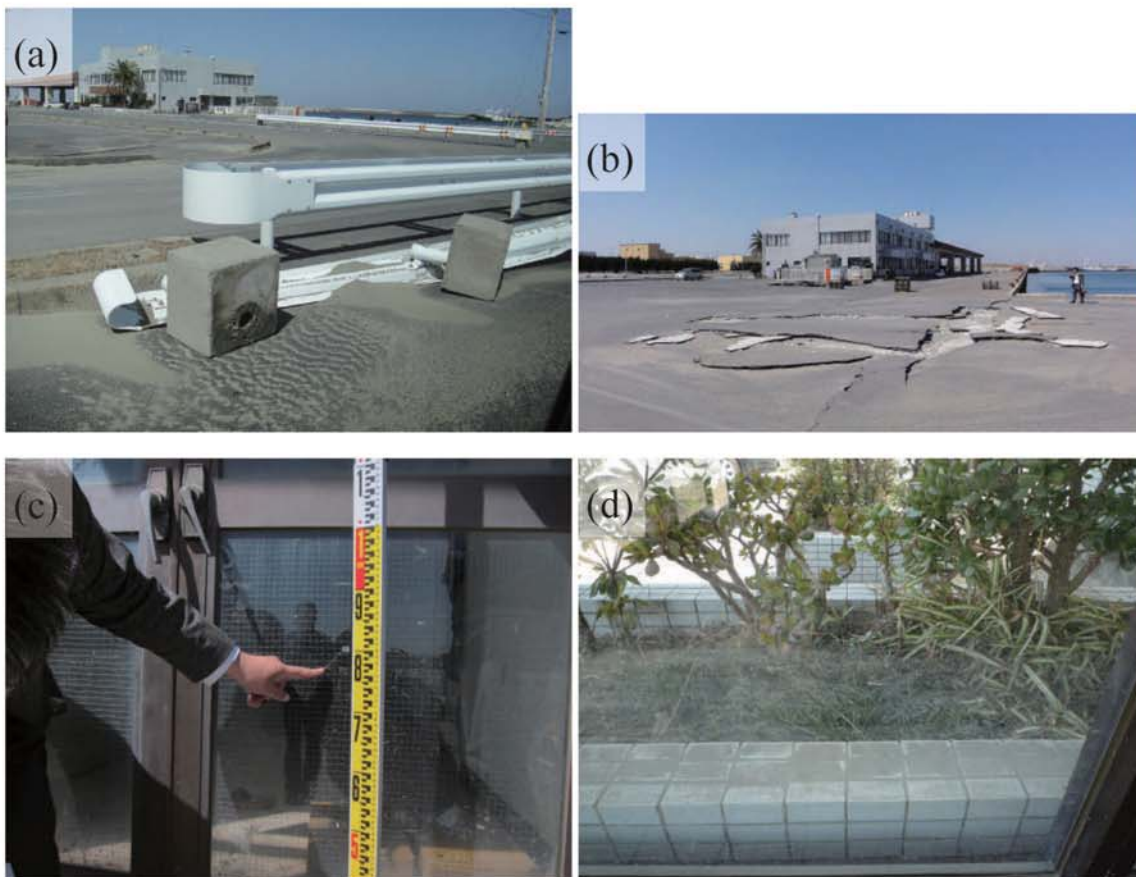
Fig. A290. (a)-(b) Damage around the fishery association building in Shin Fishing Port. (c) Watermark on the entrance doors of the fishery association building (0.898 m above ground level; B36). (d) Watermark on a windowpane of the fishery association building.
