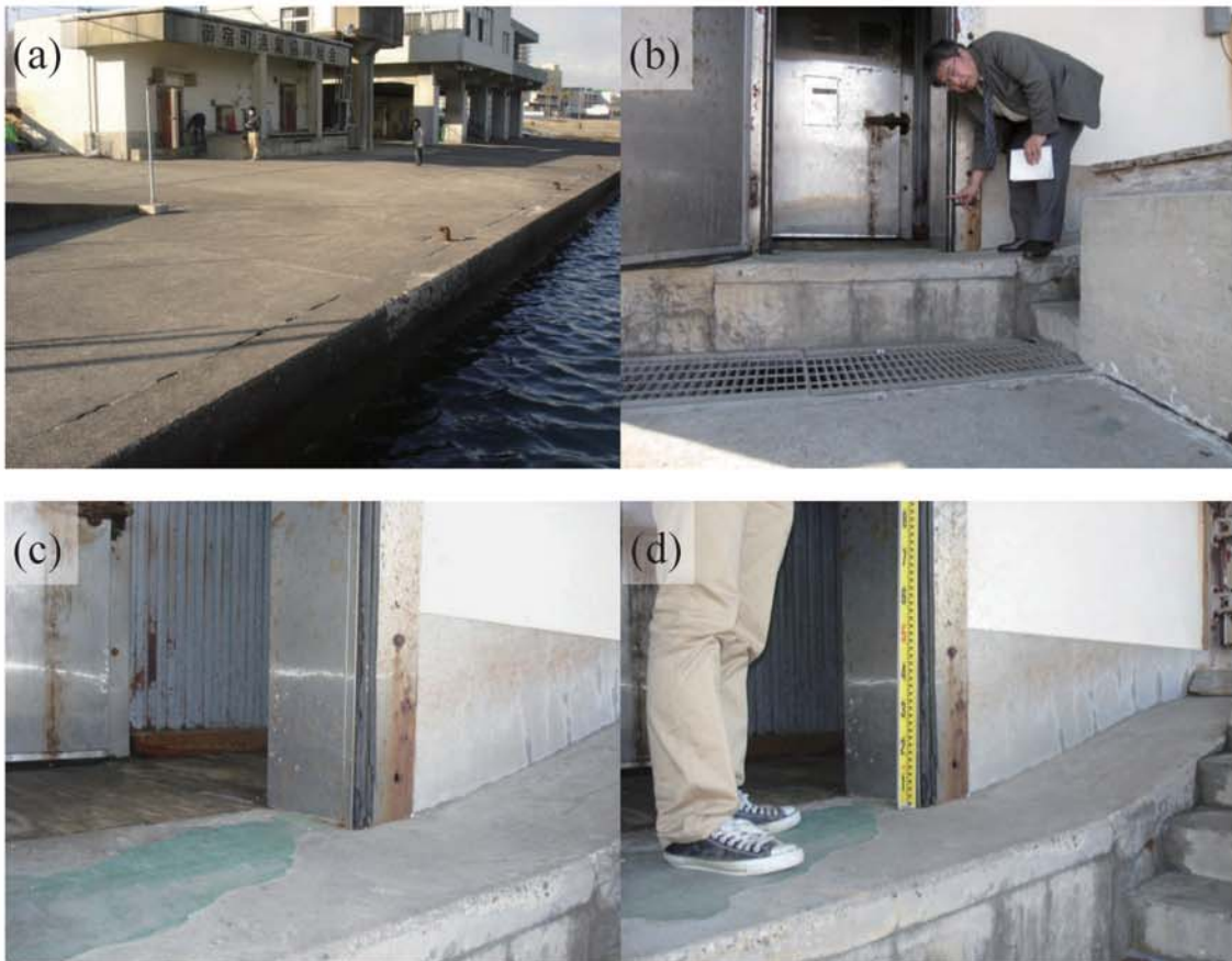
Fig. A328. (a) Freezer building in Onjuku Fishing Port. (b)-(d) Watermark on a wall of freezer building (0.305 m above floor level; C26).
