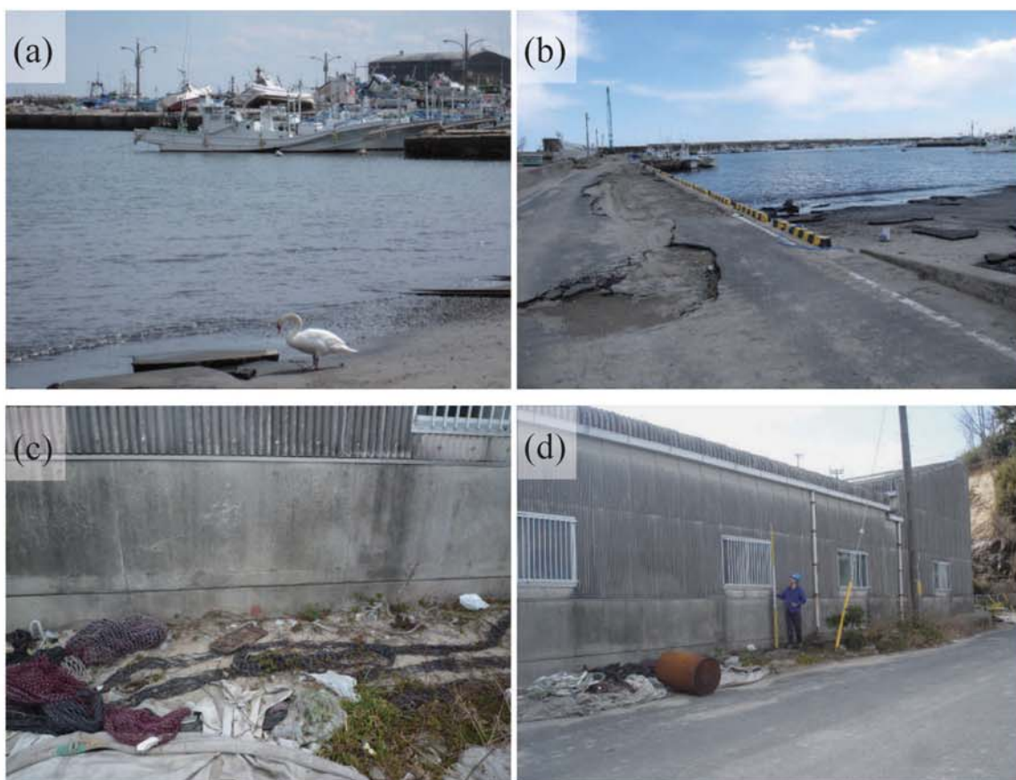
Fig. A272. (a)-(b) Damage at Kuji Fishing Port. (c) Debris and fishing nets on the road beside a warehouse in the port. (d) Tsunami inundation limit based on scattered debris (under the rod, B24).
