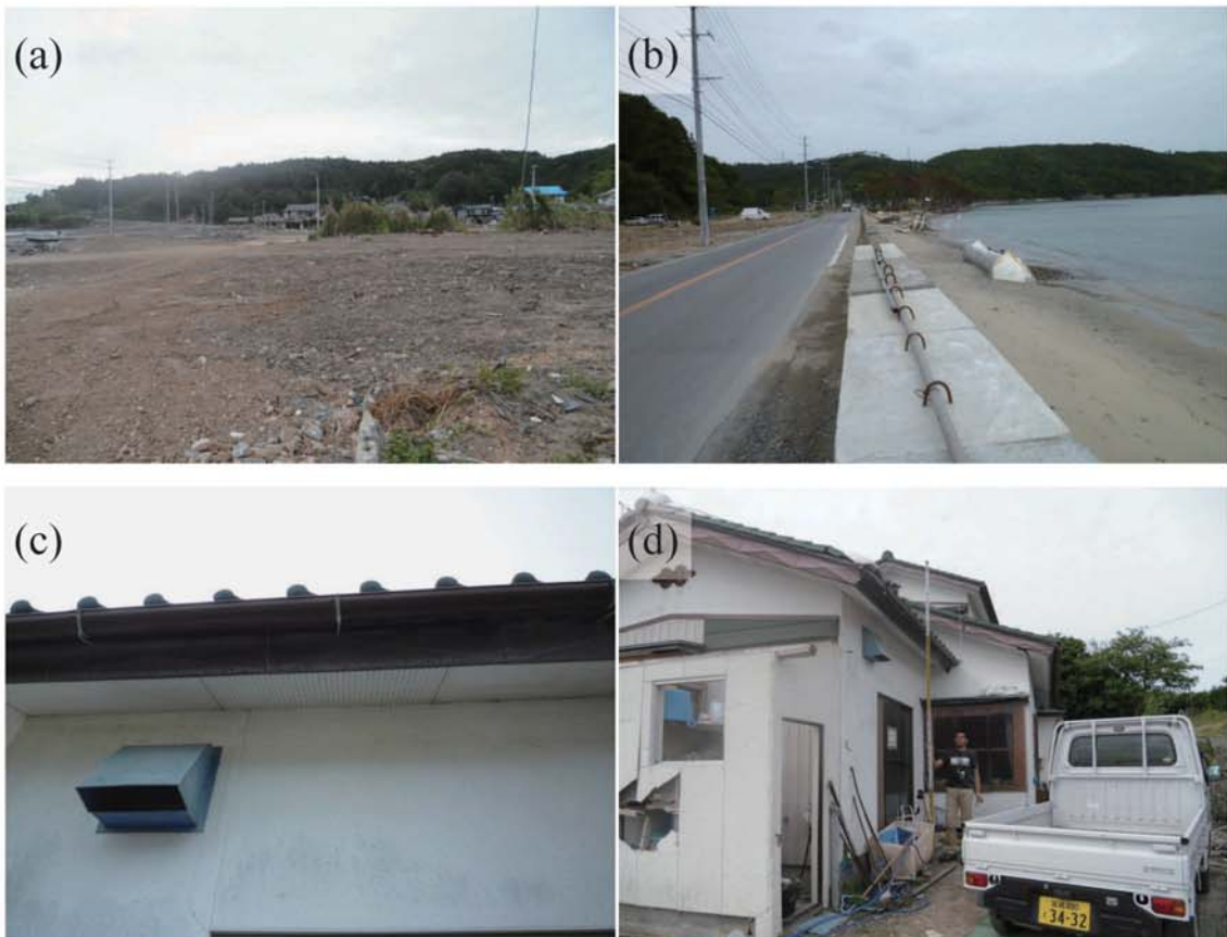
Fig. A228. (a)-(b) Damage at Kugunarihama. (c)-(d) Tsunami trace survey point on a wall of Mr. Sato's house (3.10 m above ground level, M71).
