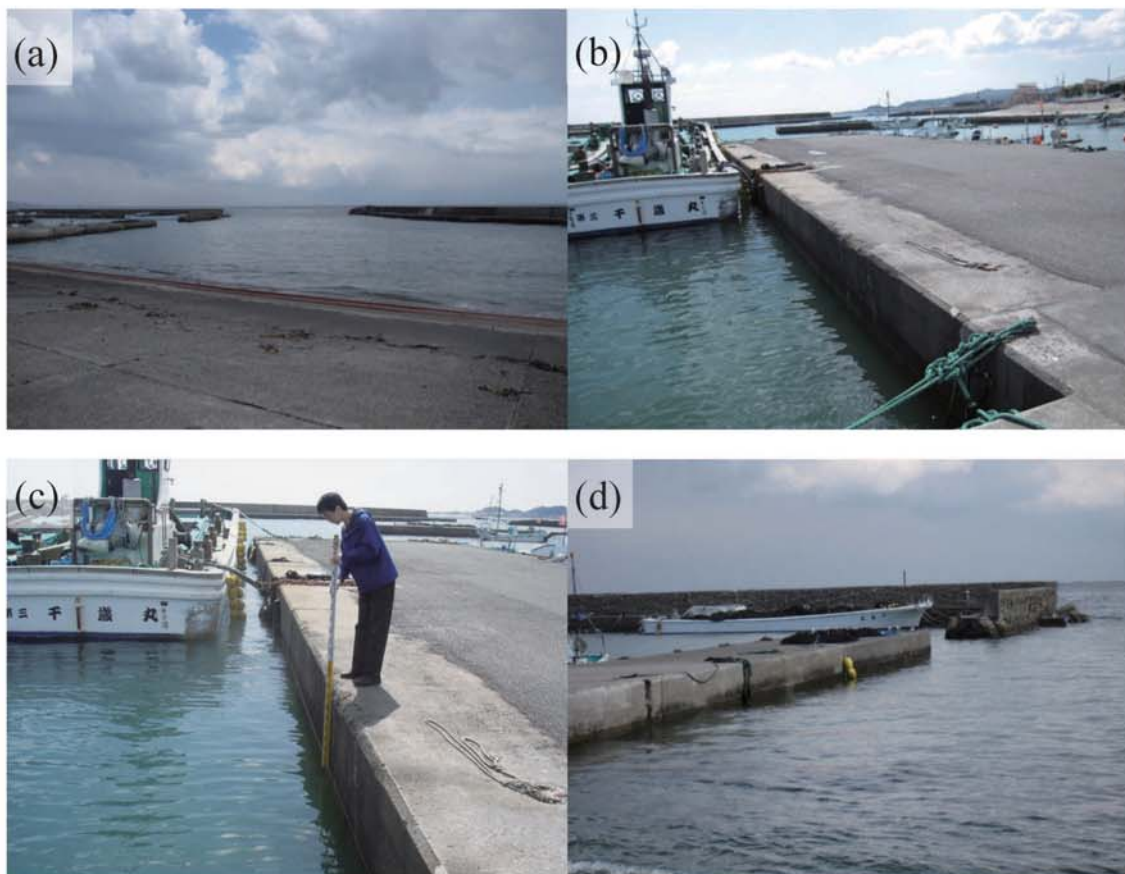
Fig. A344. (a) The Shirako Fishing Port. (b)-(c) Tsunami trace survey point at the top of a quay (C35). (d) The yellow buoys show the upper limit of the Tsunami height at the port (C36).
