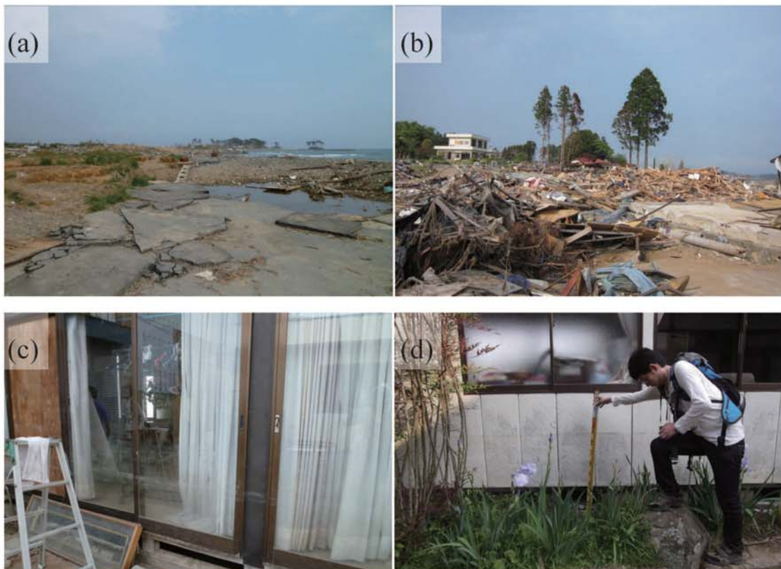
Fig. A144. (a)-(b) Damage at Hajikamisuginoshita. (c)-(d) Tsunami trace survey point on a wall of a house near Hatakeyama ironworks (0.90 m above ground level, M9).
