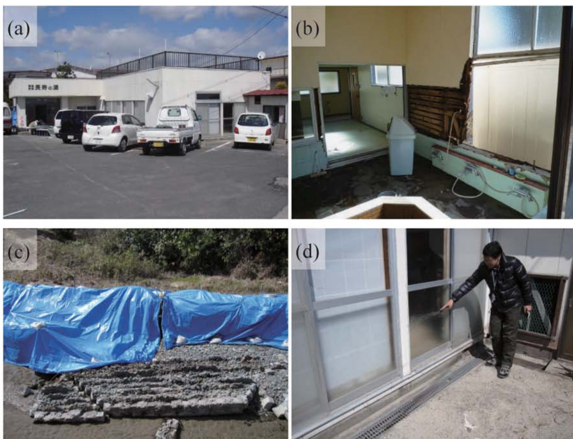
Fig. A262. (a) The spa Chojunoyu at the side of the Kita River in Higashinamekawacho (tsunami trace survey point). (b) Damage at the bathroom of the spa Chojunoyu. (c) Damage to riverside walls caused by the tsunami flowing backward in the Kita River (testimony of spa staff). (d) Watermark on windowpanes of the spa Chojunoyu (0.89 m above ground level, B17).
