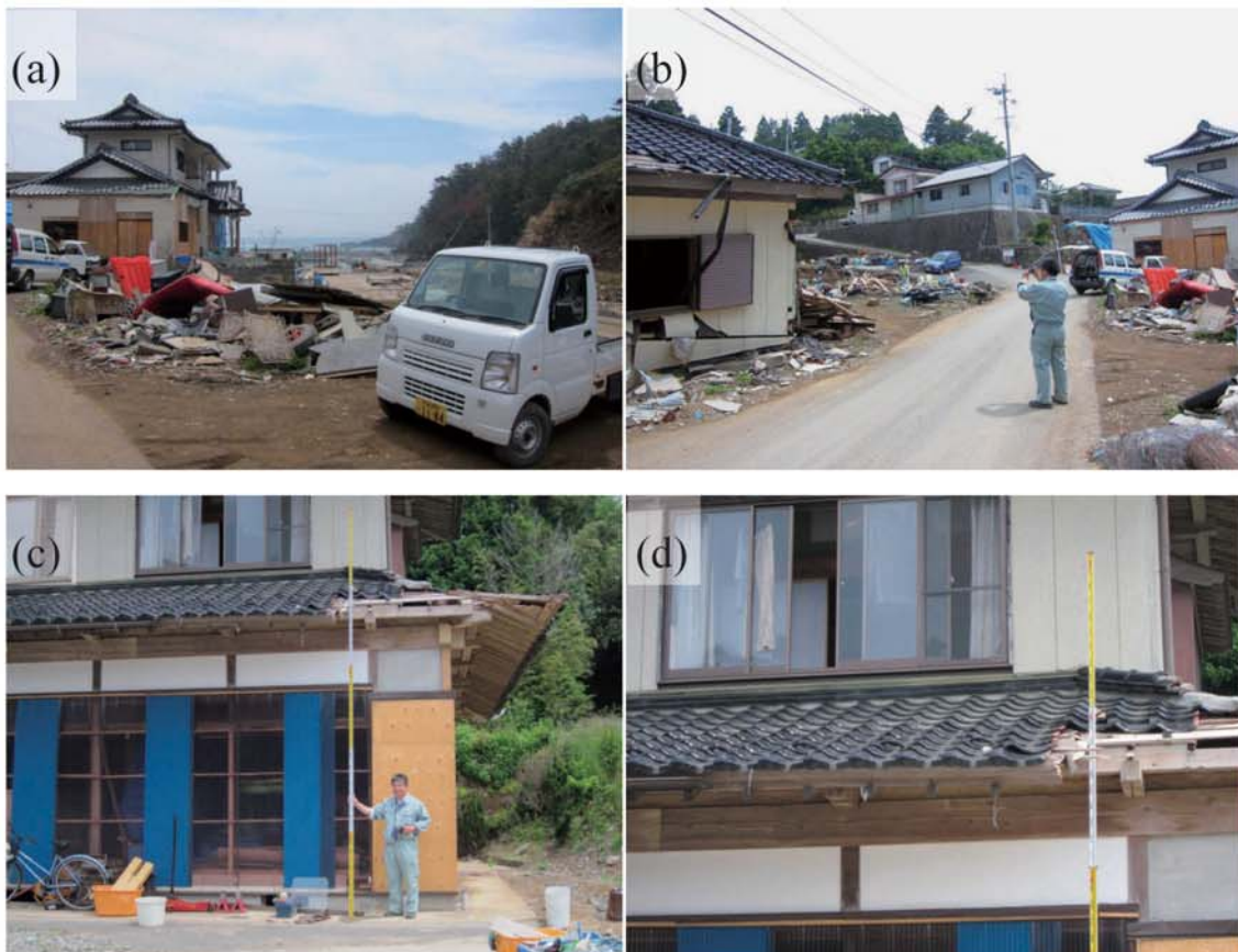
Fig. A160. (a)-(b) Damage at Utatsu-Ishihama. (c)-(d) Tsunami trace survey point on the the roof of Mr. Abe's house (4.10 m above ground level, M25).
