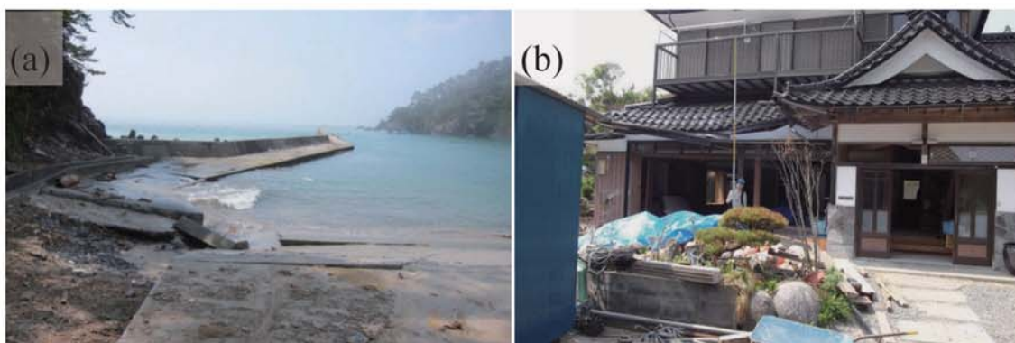
Fig. A140. (a) Damage at Karakuwacho-Tsumoto. (b) Tsunami trace survey point at the drying area on the second floor (4.7 m above ground level, M4).
