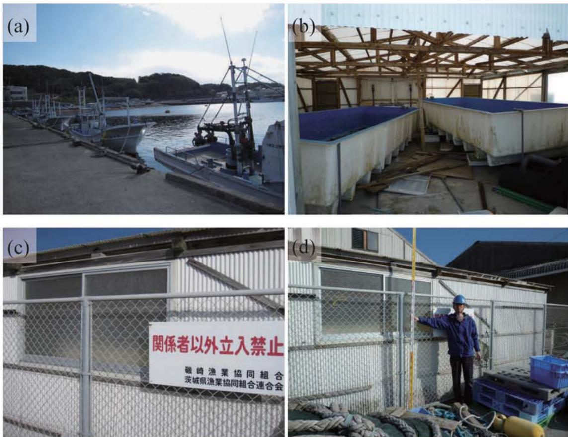
Fig. A278. (a) Isozaki Fishing Port. (b) Damage to shed in Isozaki Fishing Port. (c)-(d) Watermark on windowpanes of shed at the port (1.76 m above ground level, B27).
