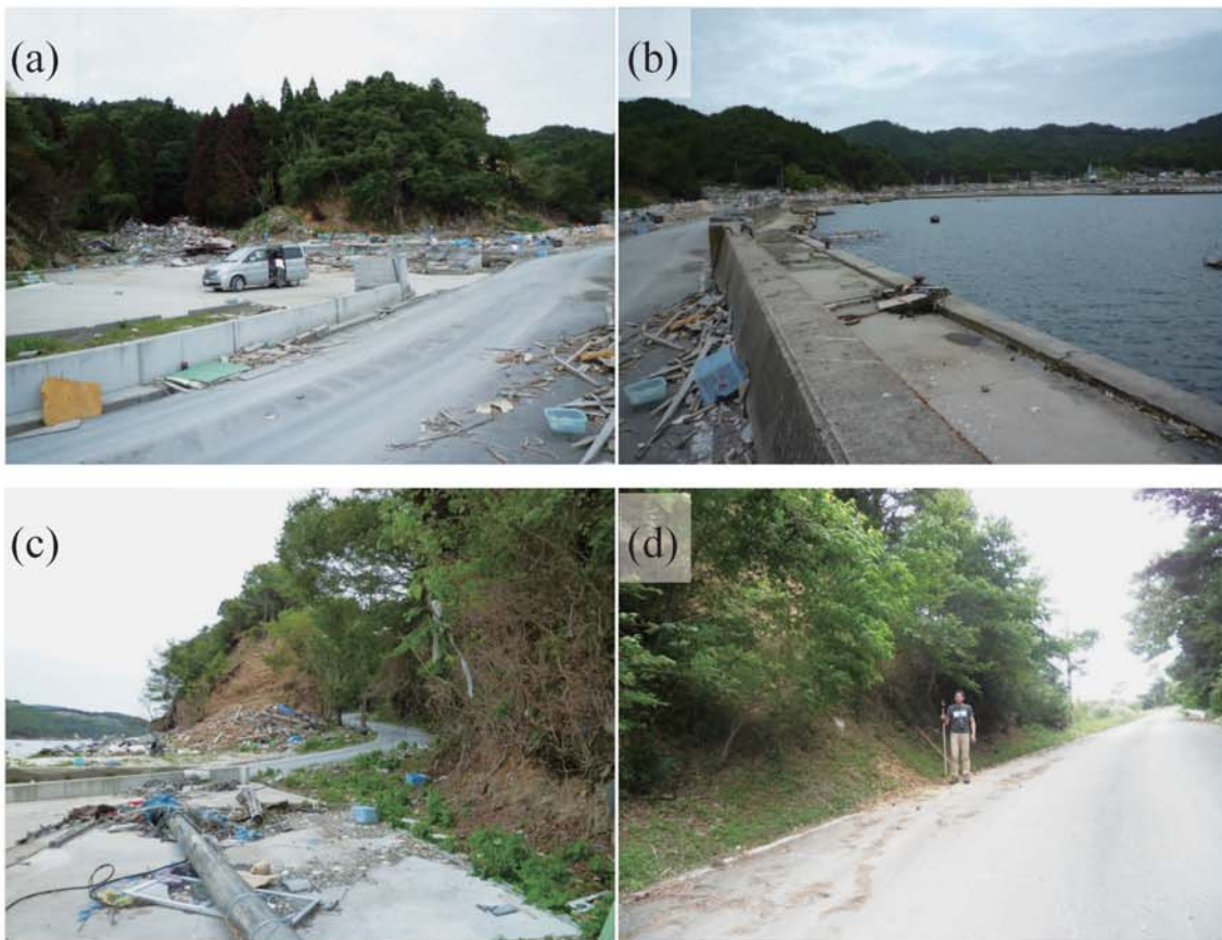
Fig. A230. (a)-(c) Damage at Koamikurahama. (d) Tsunami trace survey point at a slope (M72).
