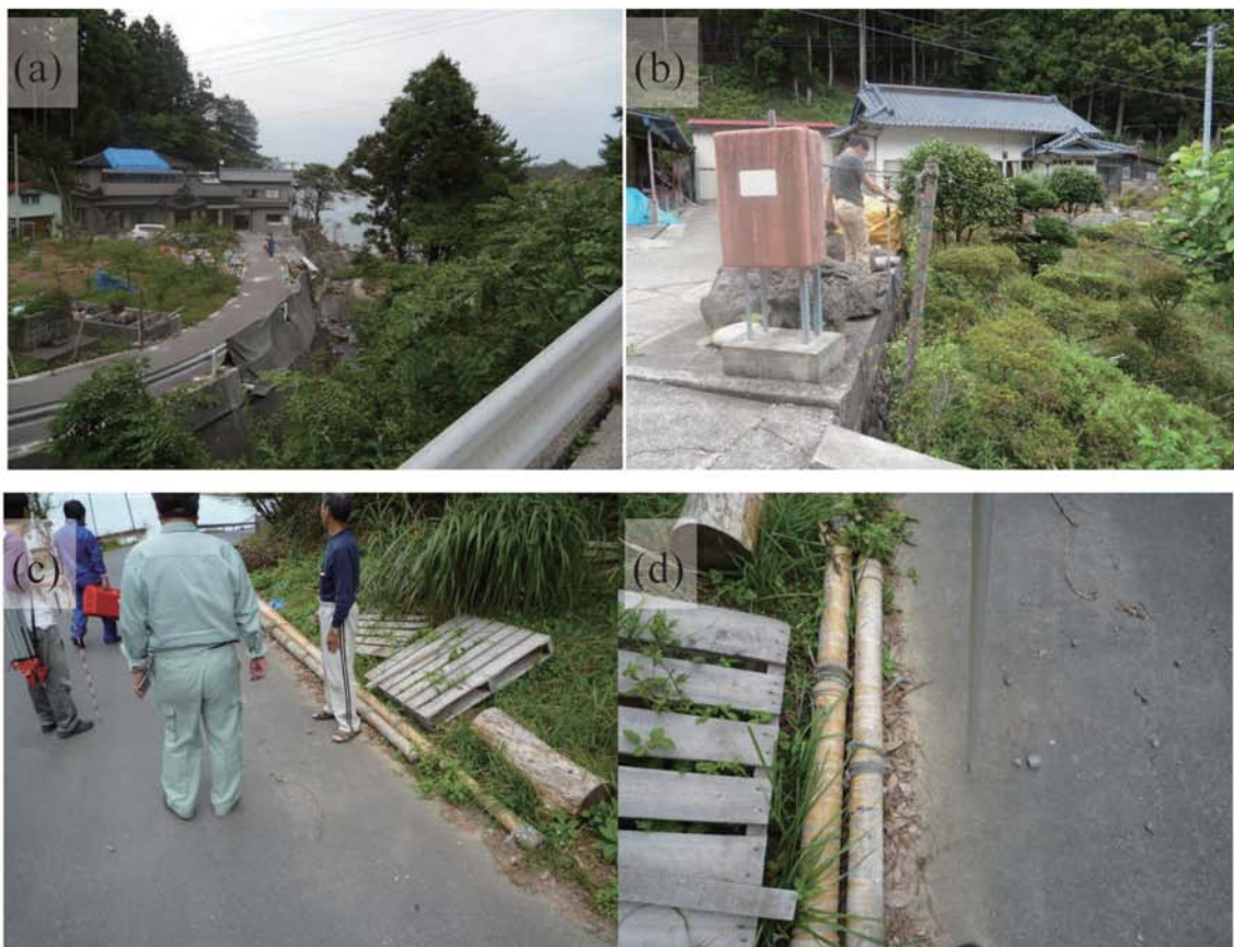
Fig. A226. (a) Damage at Tomarihama. (b) Tsunami trace survey point on the slope (M69). (c)-(d) Tsunami trace survey point on the slope (M70).
