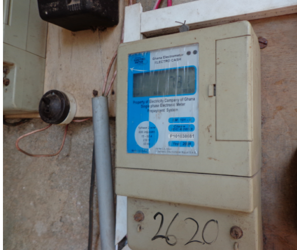
Figure 7-8: Electric power meter used in households
