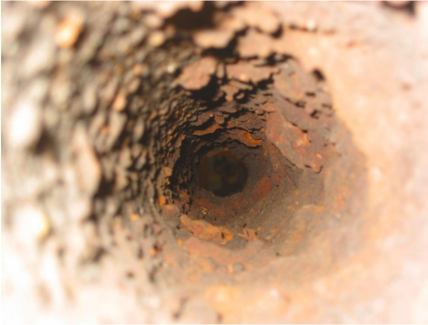
Figure 1: Photograph inside of a 4-inch cast iron pipe tested for this study
