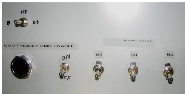
Figure 2.14: Junction box front panel.
