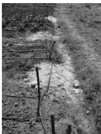
Fig. H.23. Poorly staked submain. SDS.
