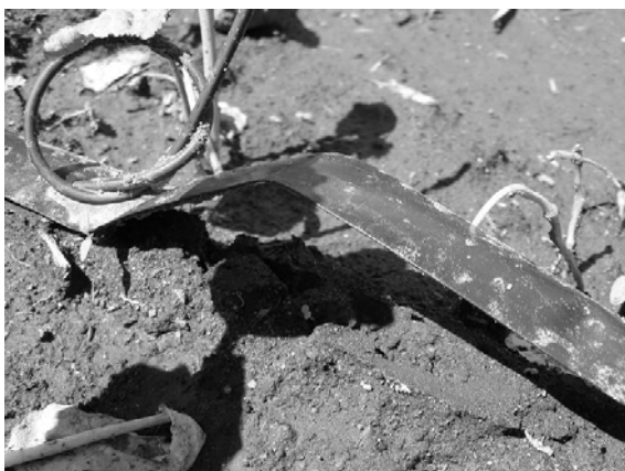
Fig. H.13. Kink in lateral from expansion due to heat/sunlight. EC3.
