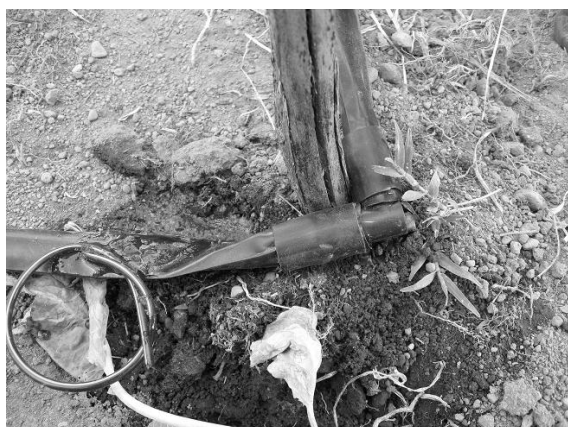
Fig. H.41. Lateral at end of submain kinked due to improper staking. Golba2.
