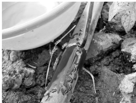
Fig. H.26. Leak at the emitter-lateral connection. AG2.
