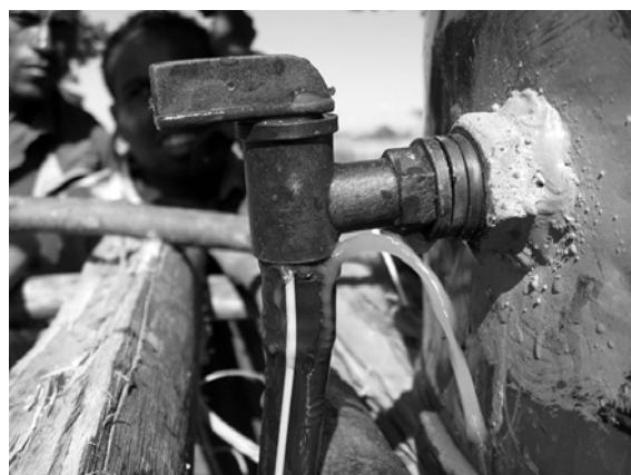
Fig. H.42. Leak at the mainline-tank tap connection. ANFTC.
