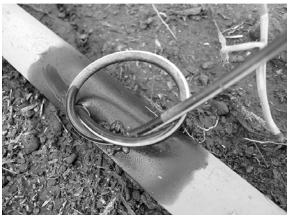
Fig. H.21. Incorrect emitter insertion. The emitter inlet points upstream, and the hole is punched off-center. DH1.
