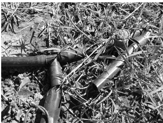
Fig. H.15. Improper submain staking. This causes a curved submain, which kinks the lateral. EC4.
