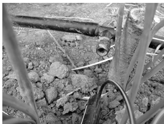
Fig. H.10. Lateral-submain disconnection. FTC1.
