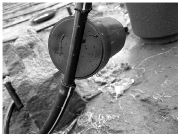
Fig. H.34. Leak in the filter casing. EC2.
