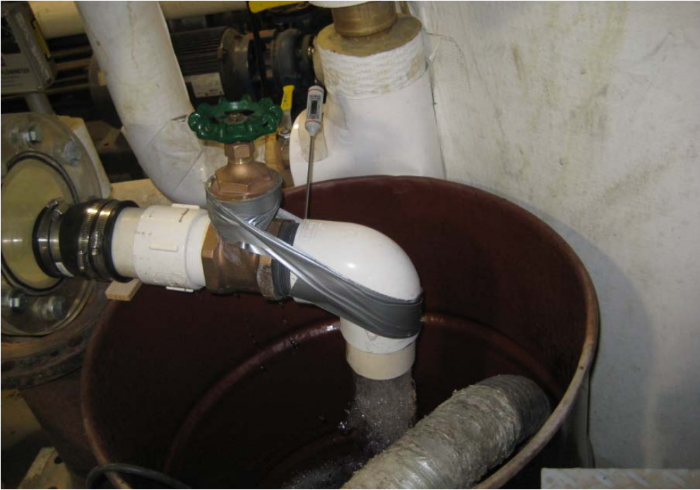
Figure 21 Downstream control valve of 3-inch pipe and thermometer for size and temperature scale tests
