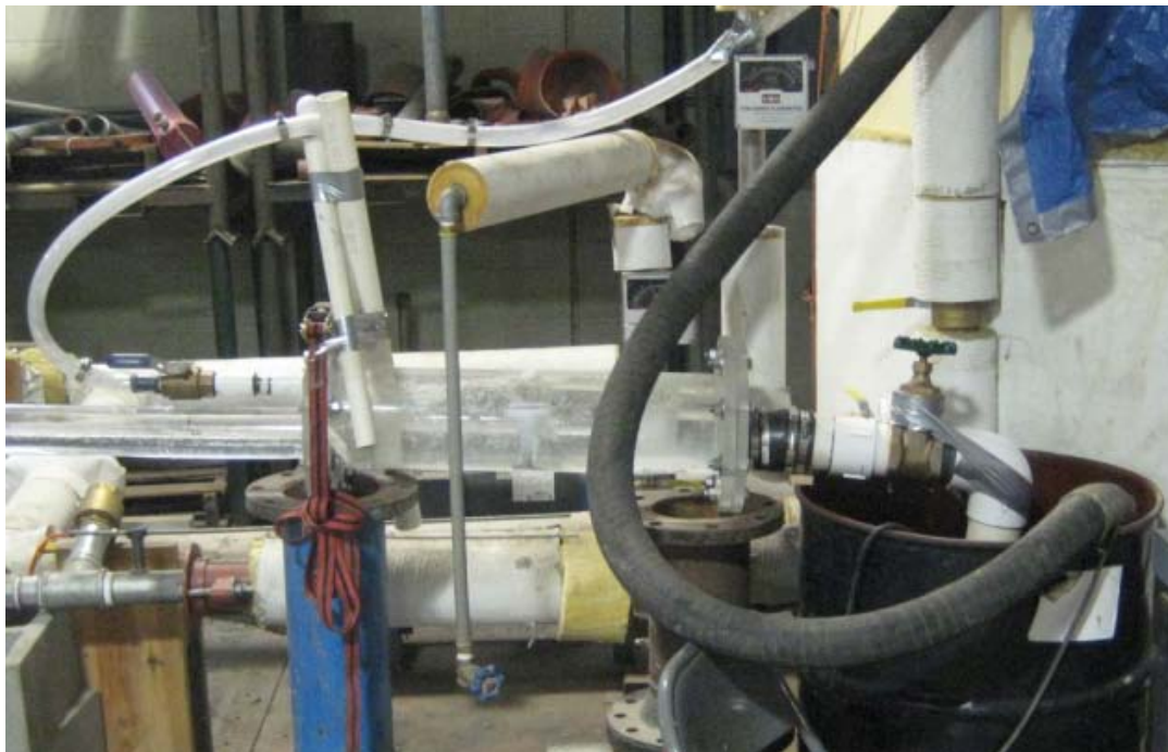
Figure 20 Air capture chamber and vent on the 3 inch acrylic pipe
