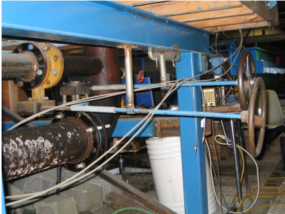
Fig. 3-7. 4-in and 8-in supply piping and orifice plates for the reservoir test facility
