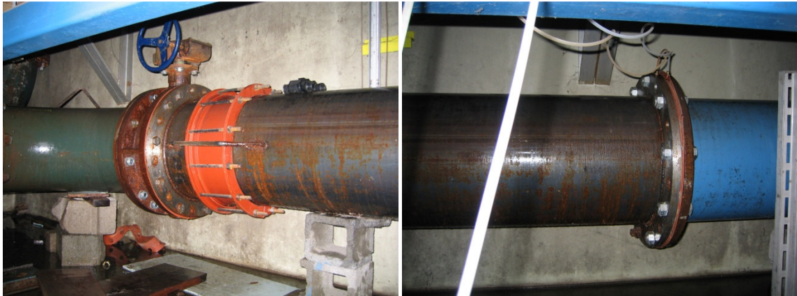
Fig. 3-8. 20-in Supply piping and orifice plate for the reservoir test facility
