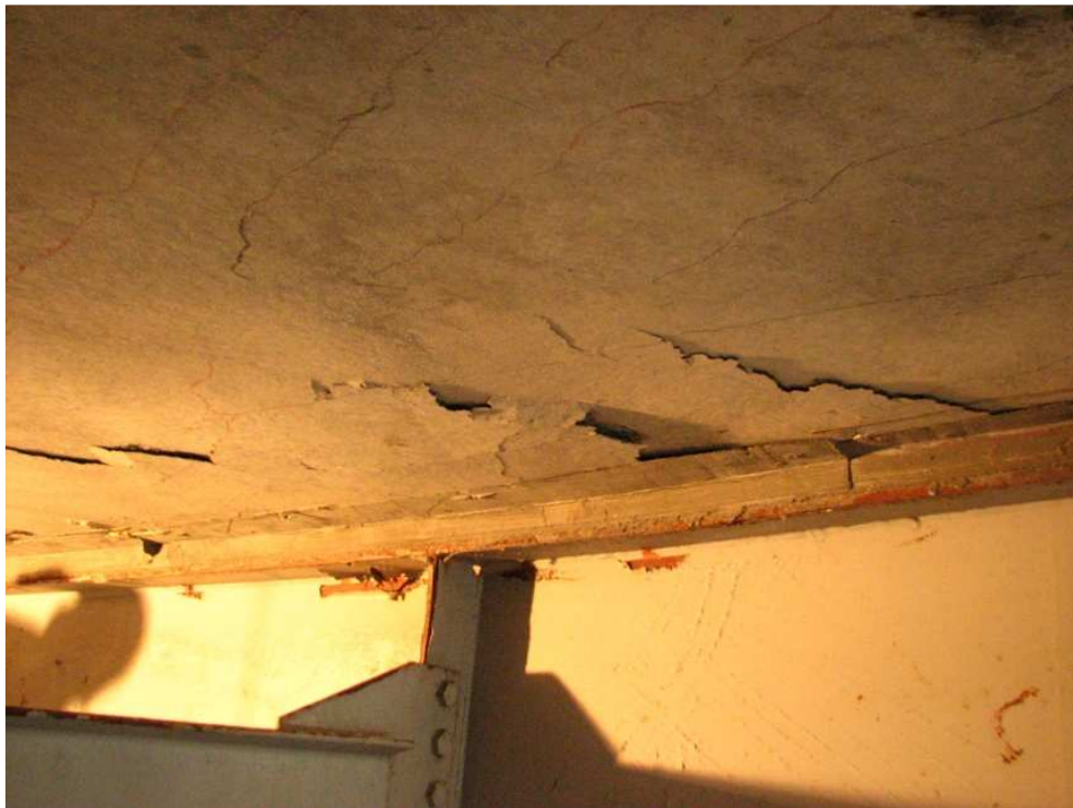
Figure 33. Delamination and Spalling Beneath Point Load at 1,420 kN (320 k ).
