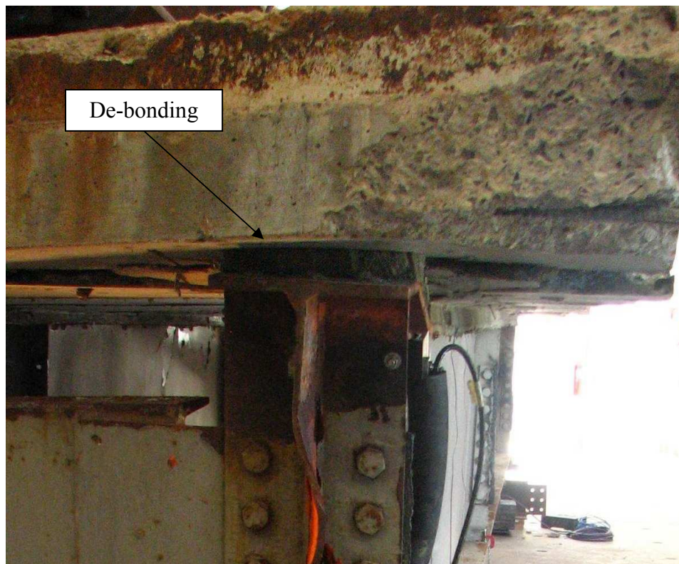
Figure 23. Grouted shear pocket failure.
