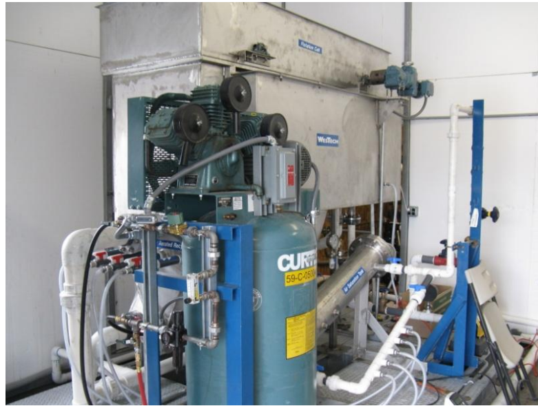
Fig. 12. Compressor and flotation tank on pilot DAF Unit
