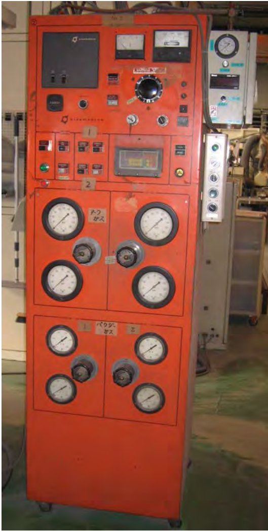
(a) Control console
