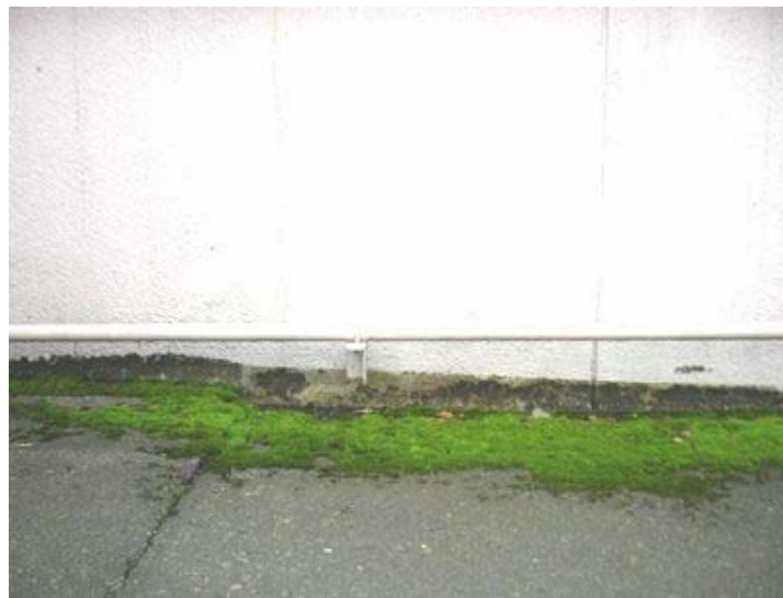
Photo 3.56- Damage caused by liquefied soil
