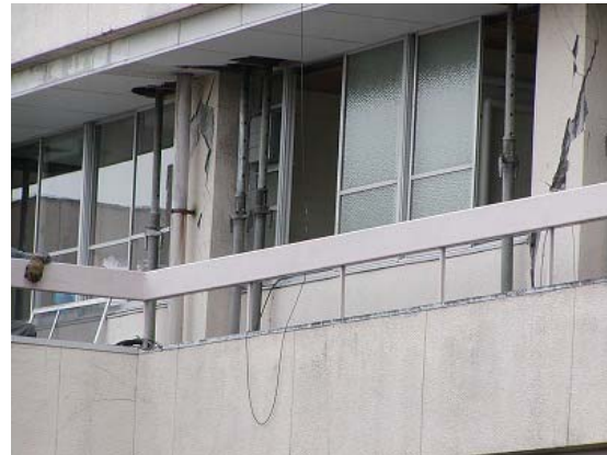
Photo 3.24- Damage to Fukaya Hospital
