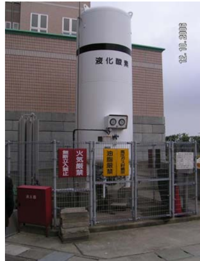
Photo 2.4- Gas supply cylinder
