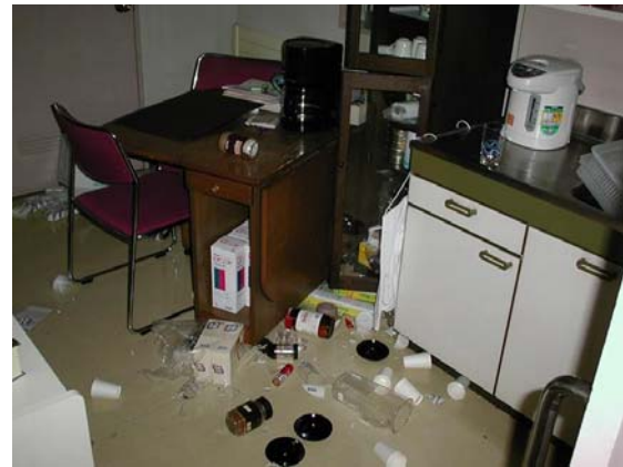
Photo 3.20- Toppling and damage to small equipment, Kushiro Urinary Clinics
