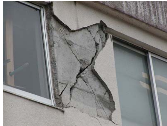
Photo 3.26- Damage to Kashimadai hospital
