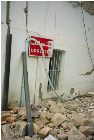
Photo 3.15- Damage to the emergency wing
