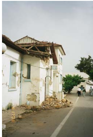
Photo 3.16- Collapsed roof of another wing
