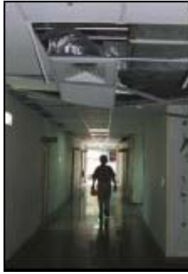
Photo 3.4-Interior damage, Veteran Hospital
