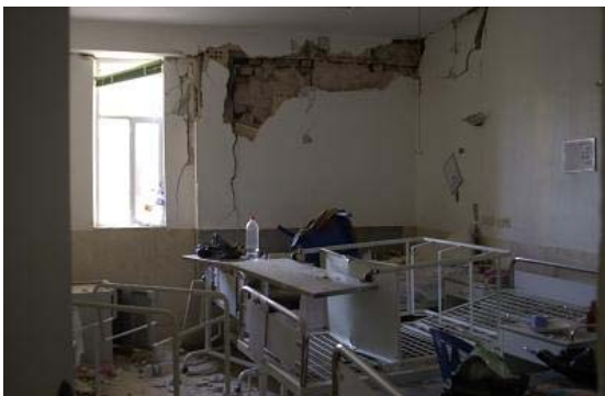
Photo 3.38- Topple of equipment Aflatoonian Hospital
