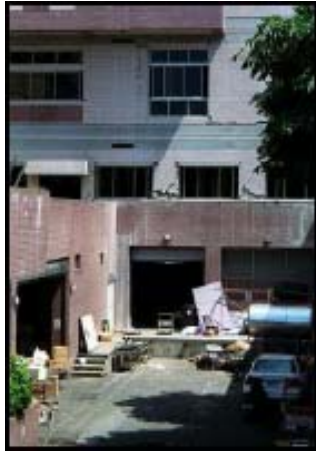
Photo 3.1- Exterior damage, Christian Hospital (Source: Lee et al, 2000)
