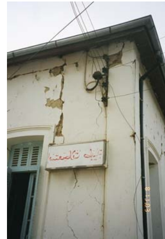
Photo 3.17- Cracks in the walls of the emergency wing
