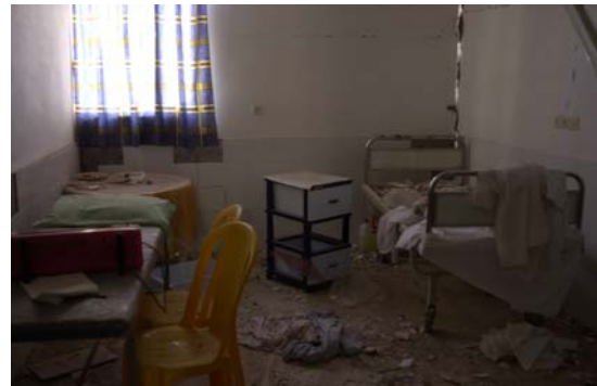
Photo II.2- Displacement of equipment
