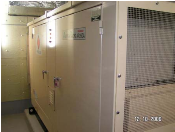
Photo 2.1- Electric power generator
