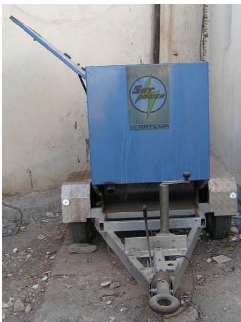
Photo 3.40- Electric power generator, Aflatoonian Hospital
