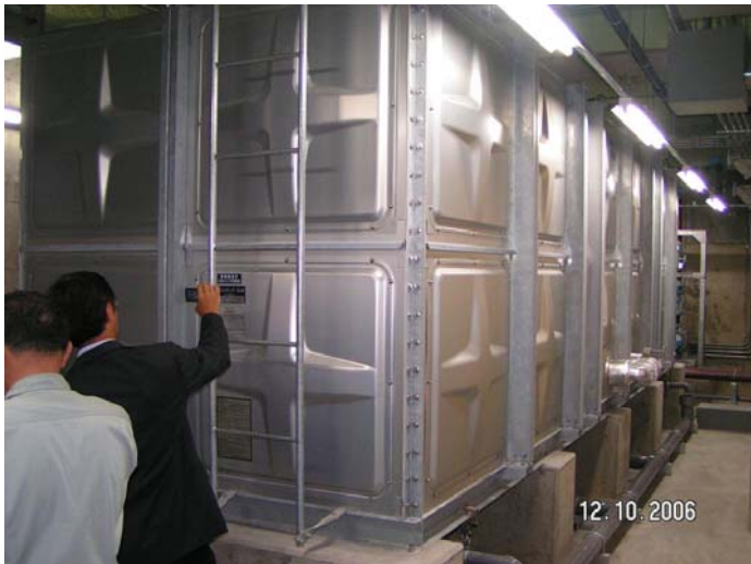
Photo 2.3- Water supply tank
