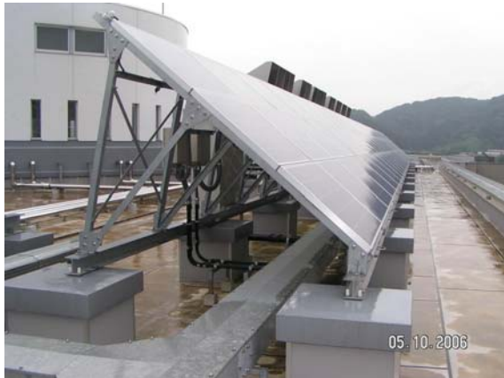
Photo 4.3- Solar panel support
