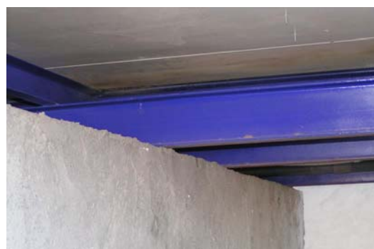
Photo 3.44- Operation room, base view
