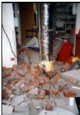
Photo 3.6-Interior damage, Shiu-Tuan Hospital
