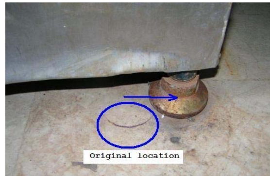
Photo 3.39- Displacement of a sterilizer Aflatoonian Hospital
