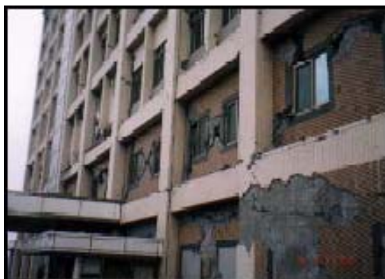
Photo 3.8- Exterior damage, Shiu-Tuan Hospital (Source: Lee et al, 2000)
