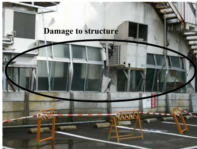
Photo 3.51- Structural damage to 1968 building, Ojiya Hospital
