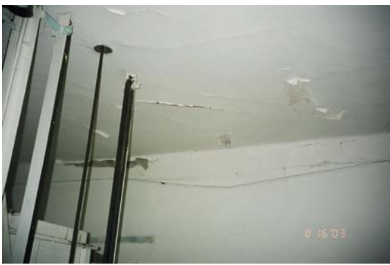
Photo 3.13- Cracks in the structure CHU Hospital
