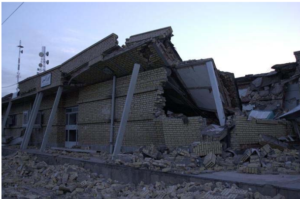
Photo 3.47- Total collapse of Imam Khomeini Hospital February 2004
