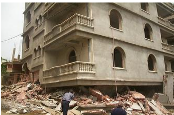
Photo 3.11- Damage to new buildings
