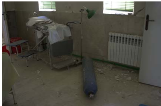
Photo II.1- Falling over of a gas cylinder
