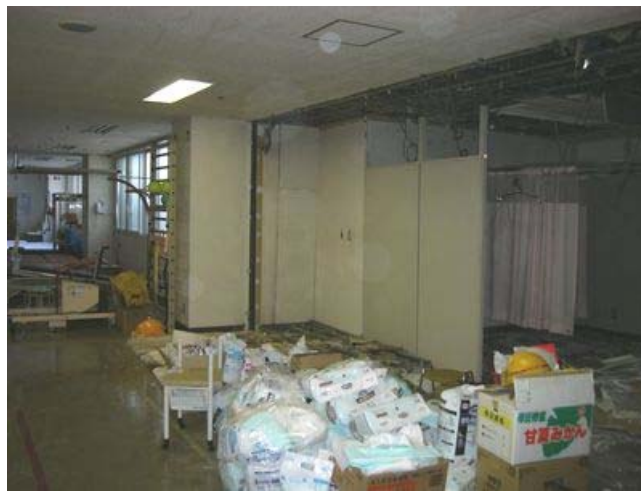
Photo 3.54- Damage to ceilings, Ojiya Hospital
