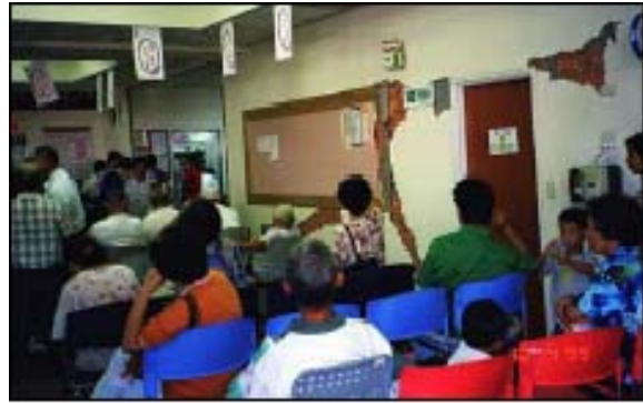
Photo 3.2- Interior damage (1 st floor, remained open) Christian Hospital (Source: Lee et al, 2000)
