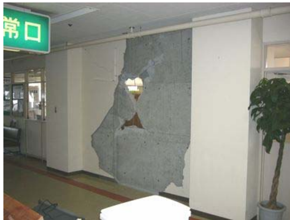
Photo 3.52- Structural damage to 1968 building, Ojiya Hospital
