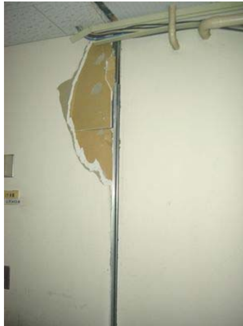
Photo 3.55- Damage to building's joint
