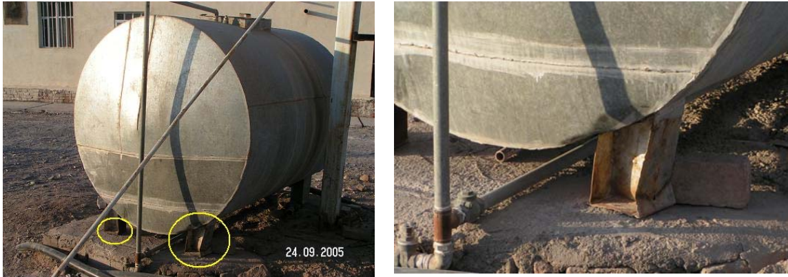
Photos 3.45, 3.46- Buckling of feet of the water tank, Aflatoonian Hospital
