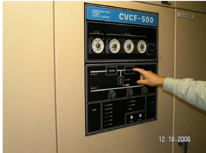
Photo 4.2- UPS control system
