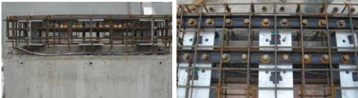
(a) Cross section (b) Plane Photo 1. Joint of the main screw re-bars and H-shaped steels
