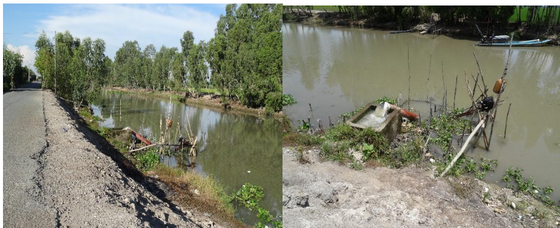
Figure 5.9: Private irrigation from a public canal into a rice field through a high dyke in the dry season at Ta Danh commune
