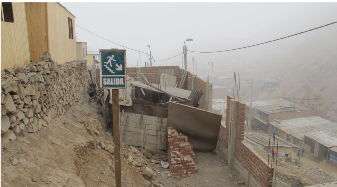
Figure 6.30: Evacuation sign pointing to a non-existent staircase and a cliff-like condition.
