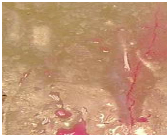
Fig. 10: Drops of water on the inside of the liner due to leakage [Bosseler 2009]
